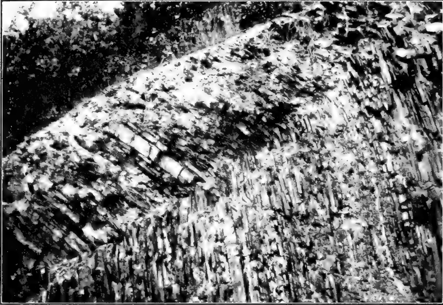
FIG. 1.—VIEW SHOWING BENDING OF ROMNEY SHALE DUE TO CREEP IN CUT OF WESTERN MARYLAND RAILROAD WEST OF TONOLOWAY.
