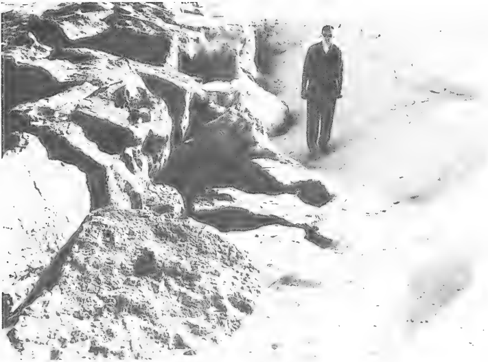
Figure 24. Damage to grouted riprap revetment at Panama City, Florida, caused by waves generated by Hurricane Hilda, October 1964
