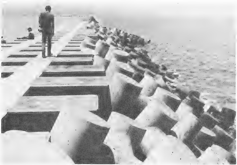
Figure 9. Rib cap on breakwater at Hilo, Hawaii
