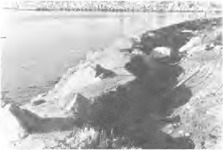
Figure 23. Damage to a grouted riprap revetment at New London, Connecticut, caused by waves generated by Hurricane Gloria, September 1985
