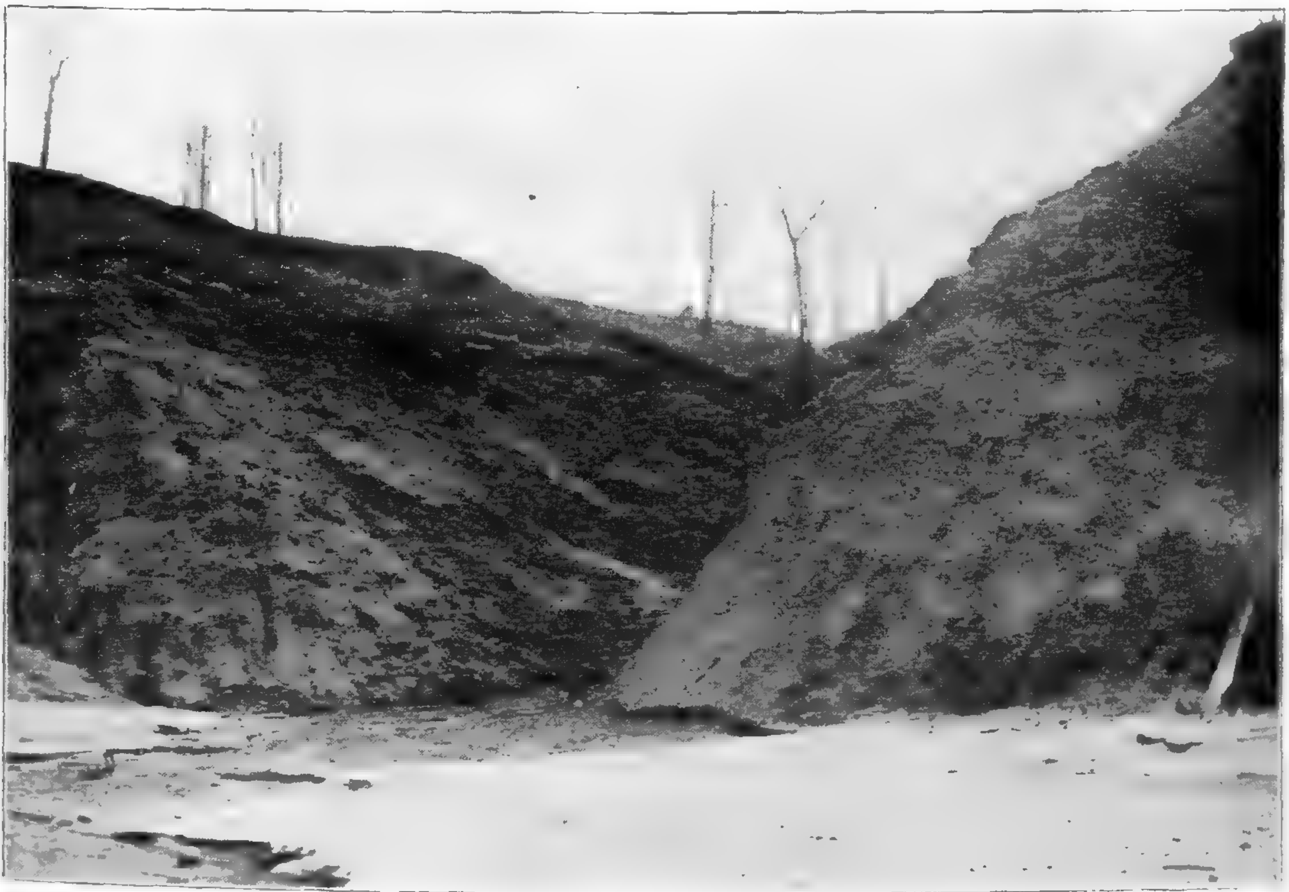
FIG. 1.—Embryonic ravine in the lake bluff at Glencoe. Entire absence of vegetation on the unstable clay slopes with the exception of shrubs and grasses that have slid down from the top.
