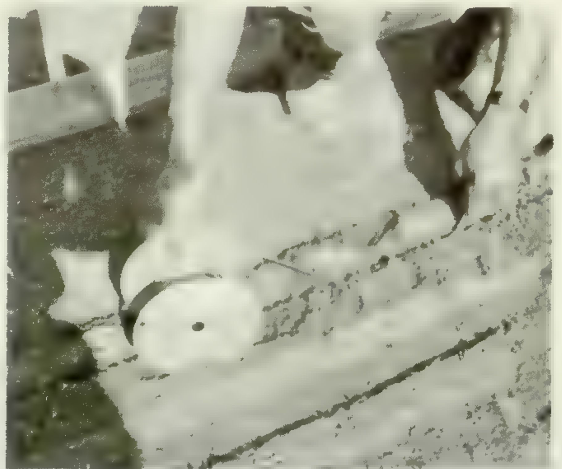
Cable being installed by hand into the trenches cut in bermudagrass sod.
