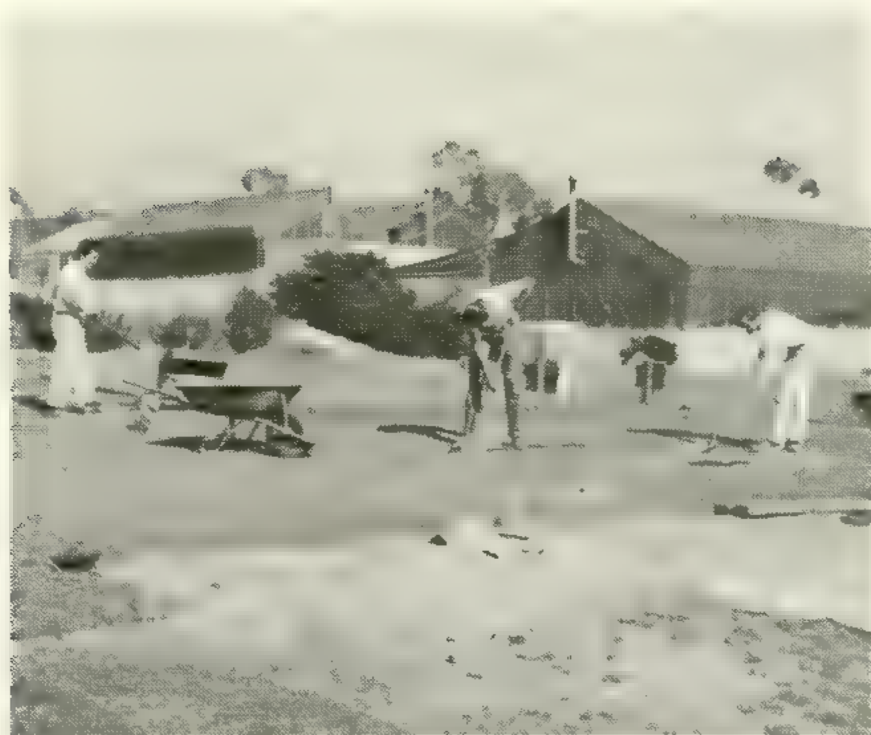
Backfilling trenches and firming soil over the cables was a tedious operation. Trenches totalled over 1/3 of a mile in length.
