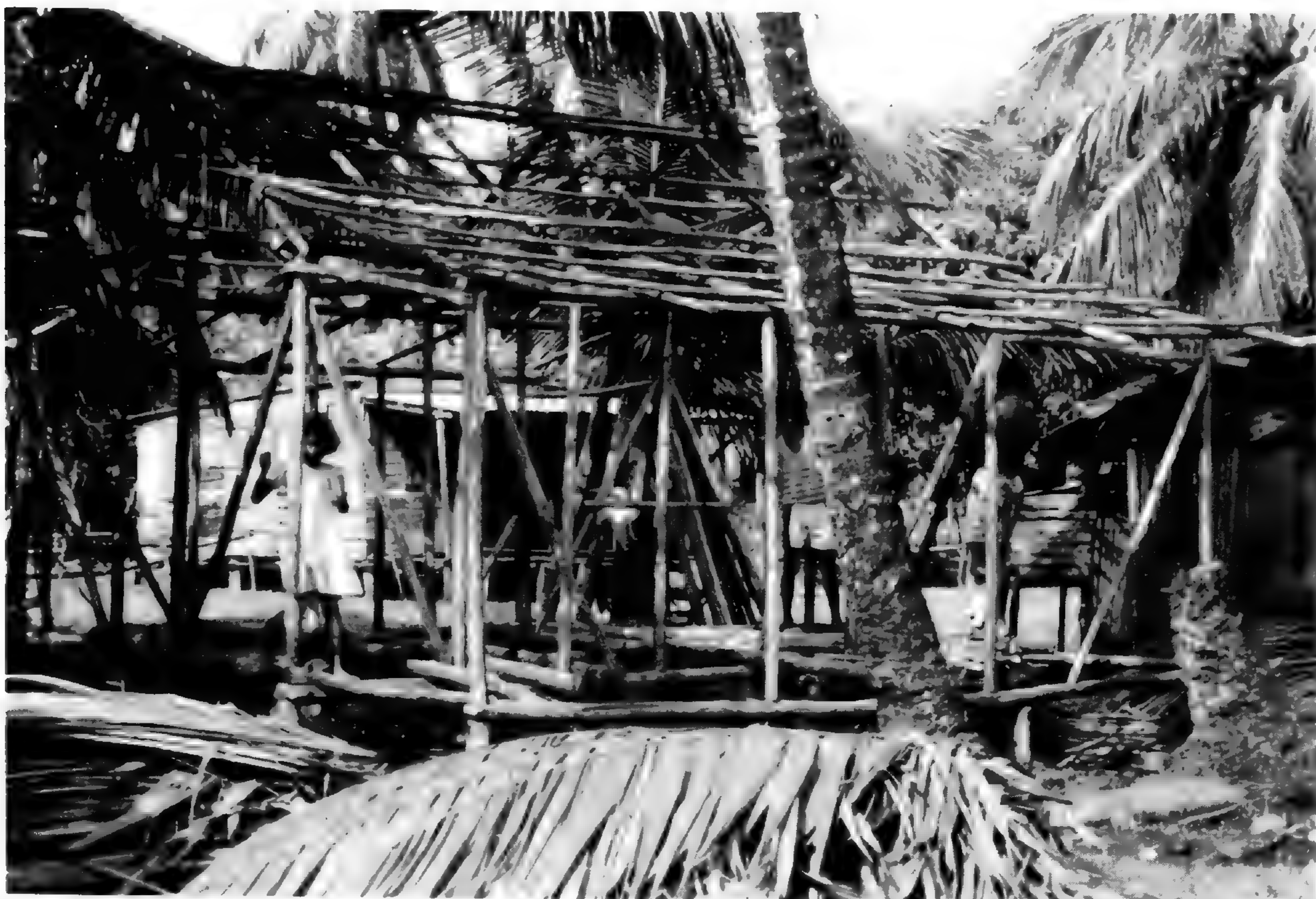
FIGURE 3.—Dwelling being built with traditional materials in the village of Tasbapauni (includes structural logs of leche amarilla, samu [ Symphonia globulifera ], and thatch of American oil palm, batana [ Elaeis oleifera ]).
