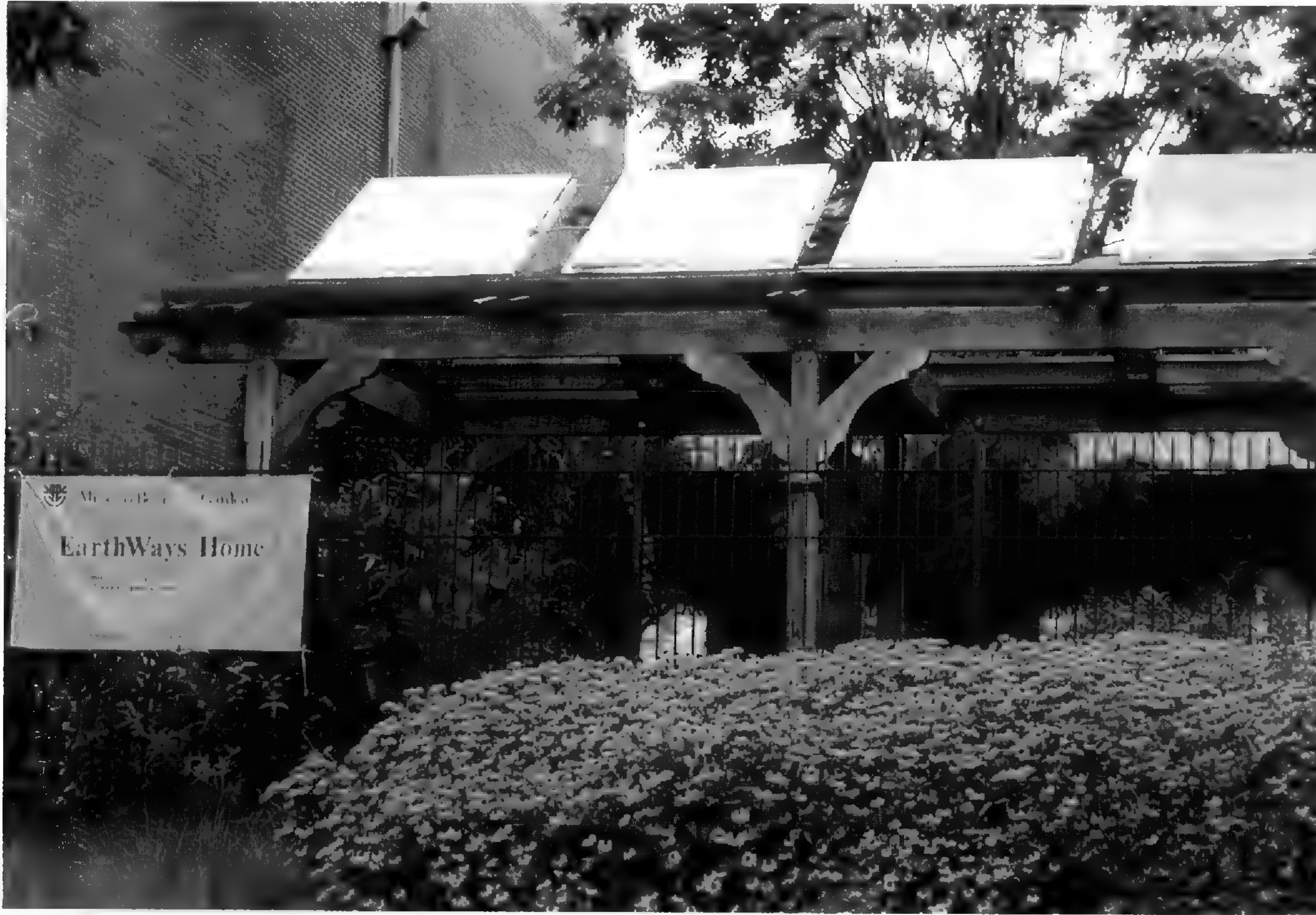
A south-facing garden pergola holds solar panels that generate electricity for the EarthWays Home.
