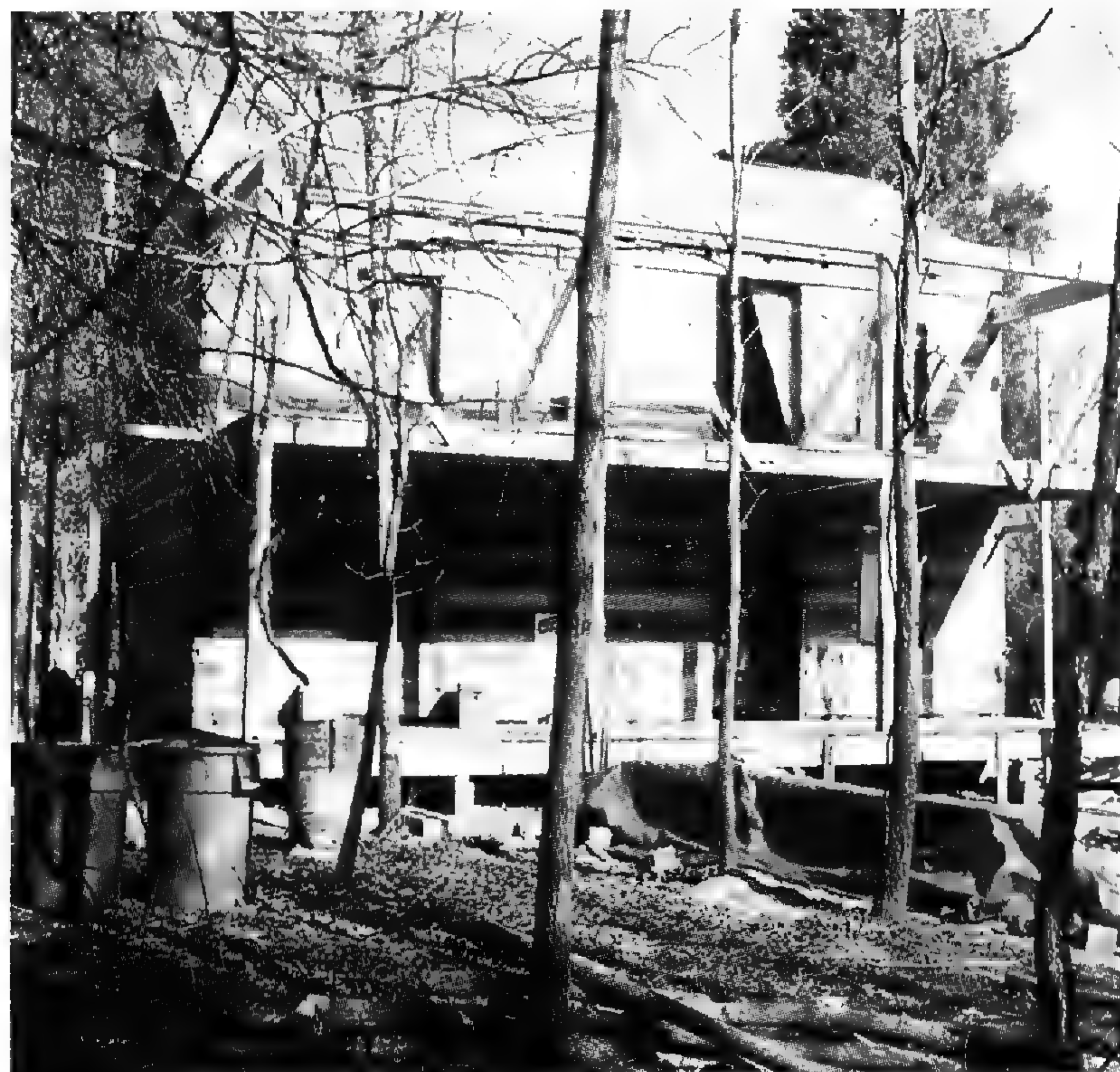
The Lichtenstein Cabin is being meticulously constructed at Shaw Arboretum using traditional craftsmanship. When the cabin is finished, it will have a two-story front porch.
