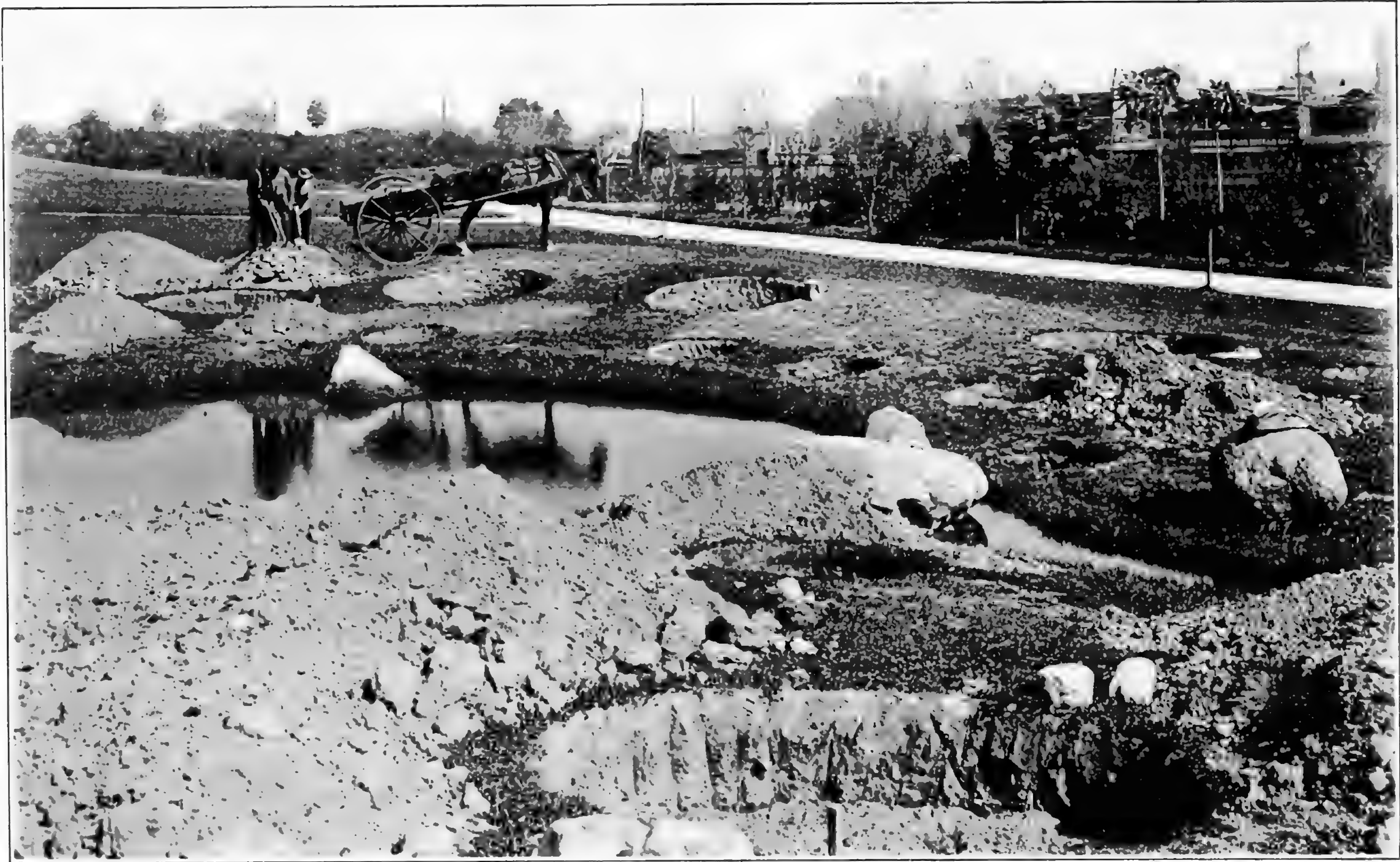
FIG. 12. Preparation for willow planting; terminal pool of the Brook, October 17, 1912. Facing east.
