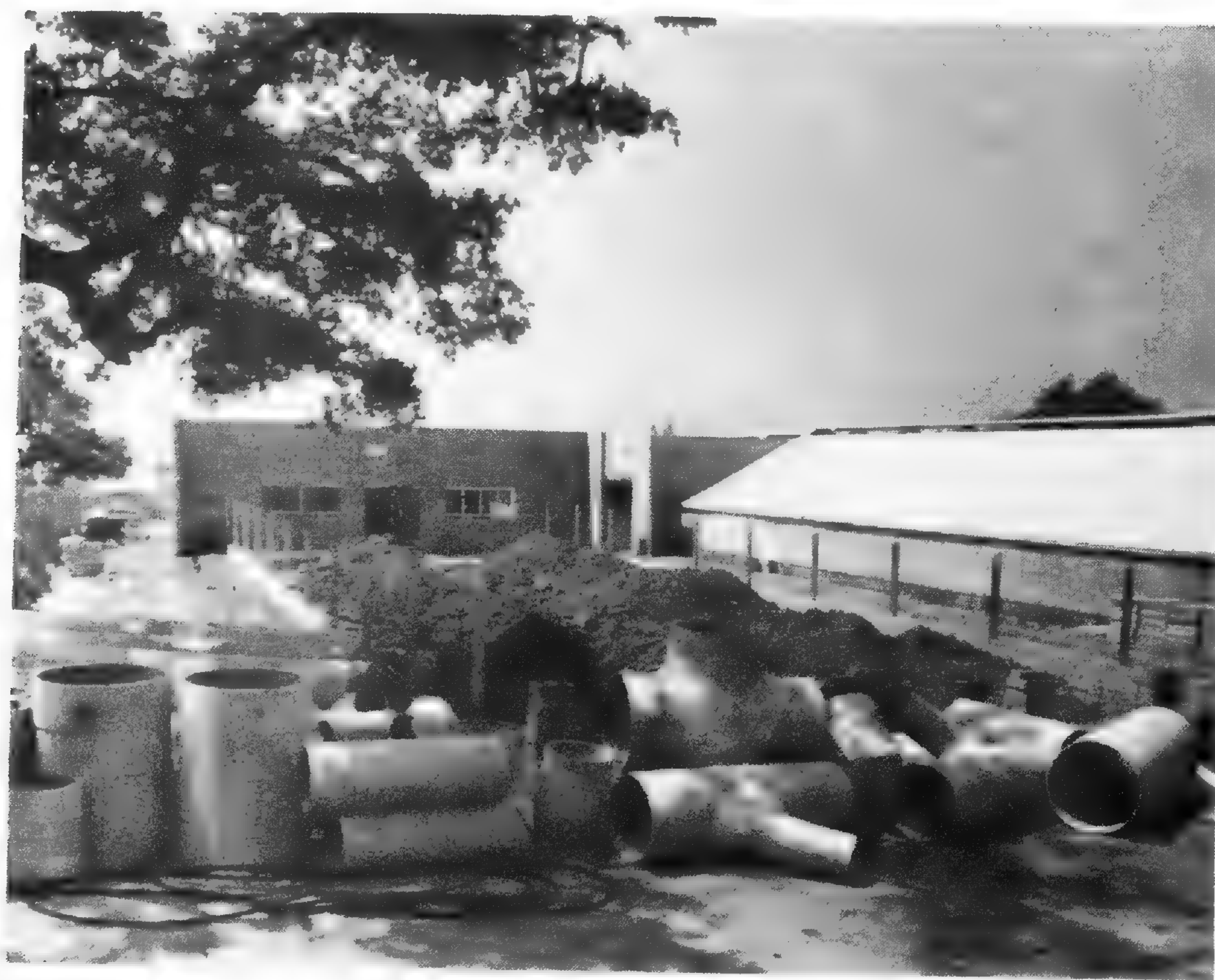
The beginnings of our second glasshouse. Office facilities will be located in the concrete block headhouse at the far end.
