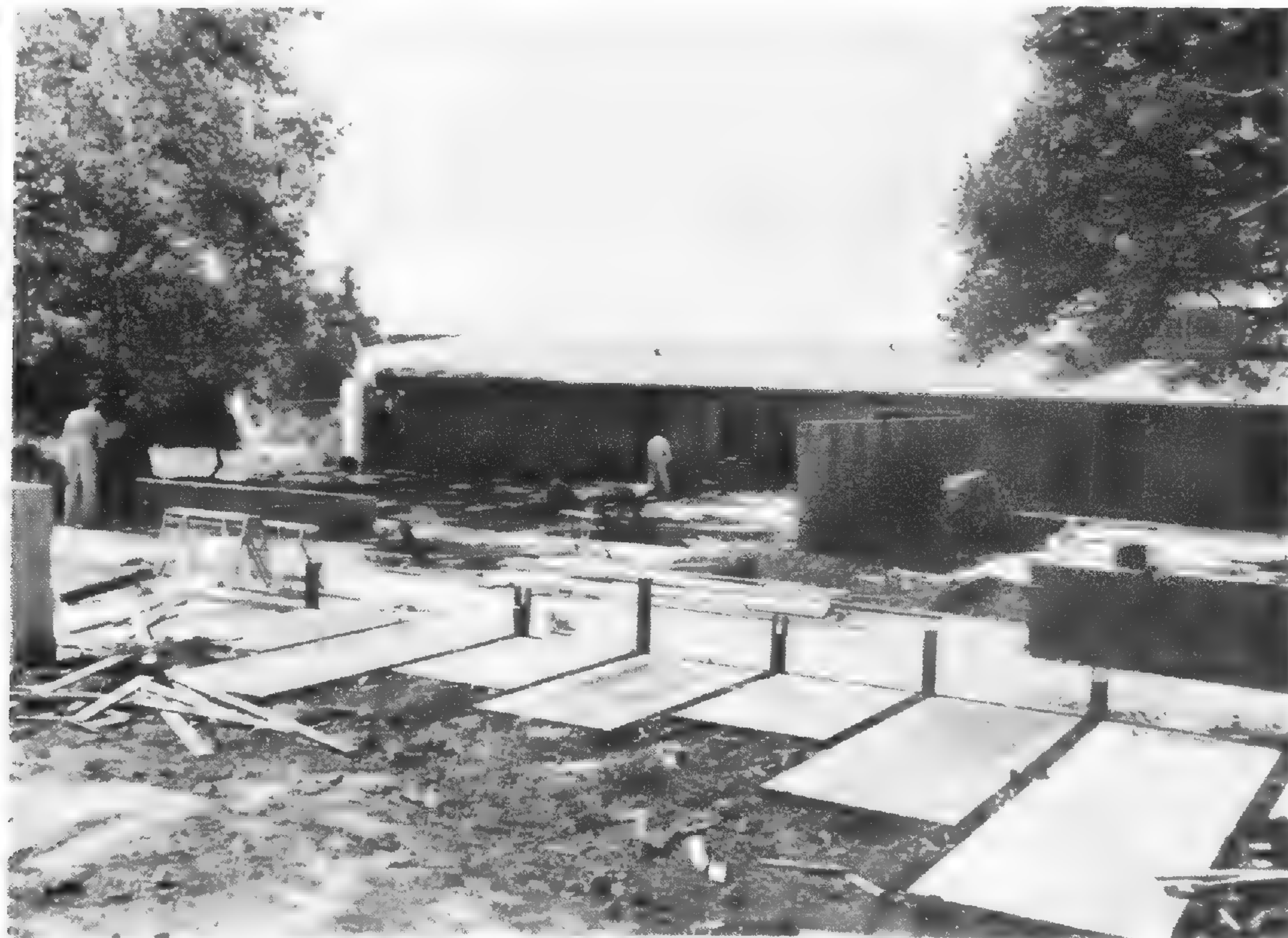
Site of the Home Demonstration Gardens north of the Administration Building. Various treatments of concrete slab surfaces are visible in the foreground.
