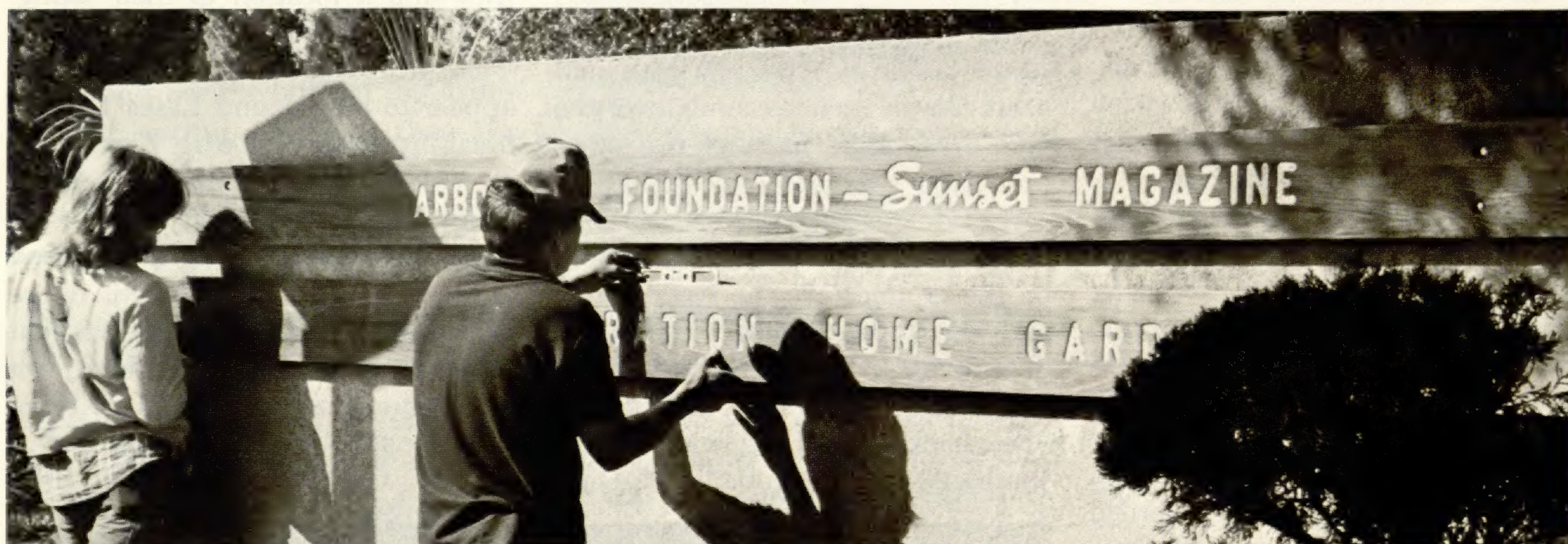
A new redwood sign goes up, welcoming visitors to the renovated garden.
