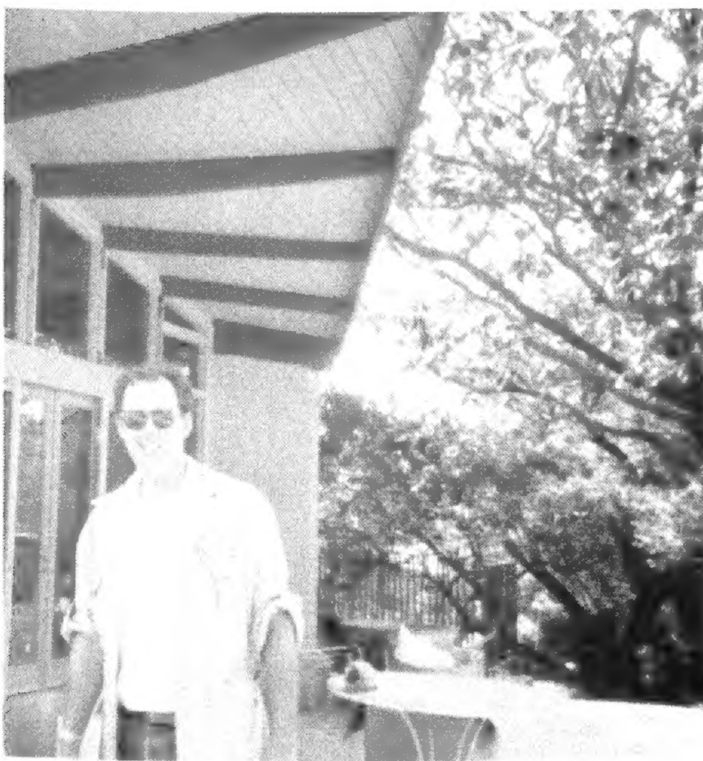
Architect Douglas Campbell of Campbell and Campbell supervises the Peacock Cafe Construction.
