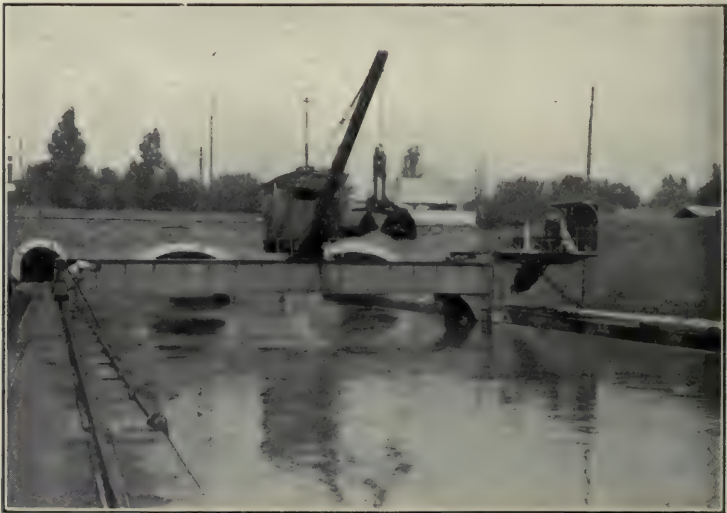
Clichy, near Paris—Settling-basin for the Sewage of Paris. Sand and other heavy, coarse matters settle and are screened here. The basin is constantly dredged. The material excavated is deposited in barges and carried to the country and spread upon land.
