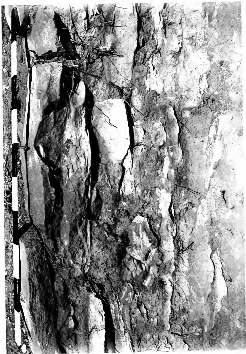
FIG. 62. Site 1, House Group I. Masonry in west wall, Room 5. Meter stick on top of wall.
