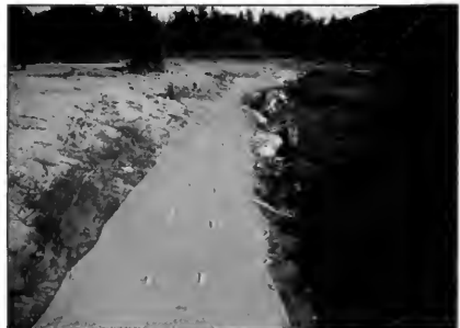
Proper installation of fabric mats is essential to success, including adequate foldover of the toe, overlap of the mats, anchoring with staples, live stakes, etc.
