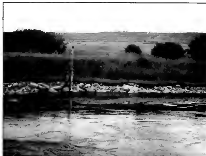
Coconut logs may be used with geotextile fiber mats for bank protection. The application above relied on a rip-rap toe to stabilize the streambank.
