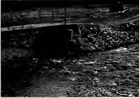
Median barriers don't usually make very good bridge abutments, or retaining walls.
