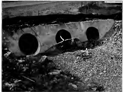
Multiple pipes are sometimes acceptable, but they can catch debris. Consider aluminum box or squash pipes.
