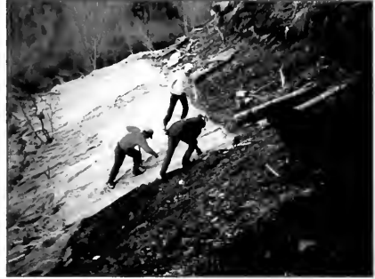
In combination with vegetation, synthetic and natural materials can provide excellent bank stability.
