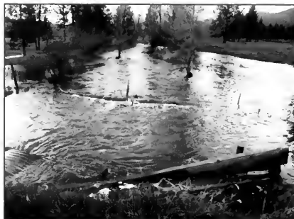
This undersized culvert caused large amounts of gravel to deposit in the channel upstream. Woody debris must be cleaned frequently from the inlet.
