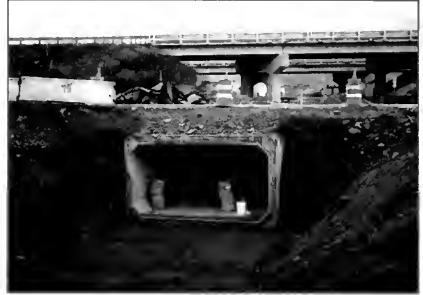
Concrete box pipes frequently have poor fish passage characteristics because of the smooth, flat bottom.
