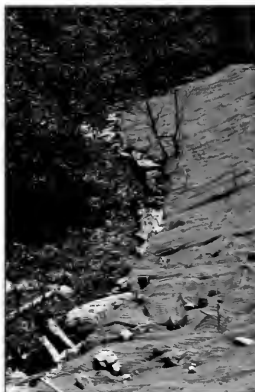
This bank treatment has a rip-rap toe but uses geotextile for the bank and is a good compromise solution.
