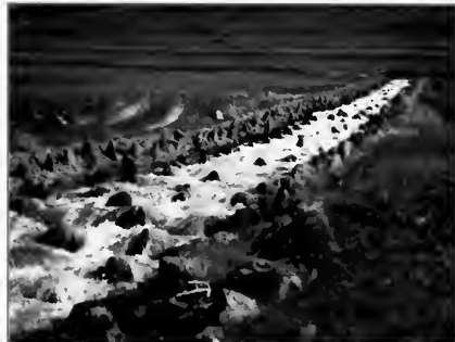
This unique drop structure is a concrete channel studded with rock to slow velocities. Structures are more commonly large rock or formed concrete.
