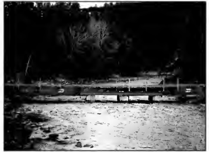
Railcar bridges are popular and fairly solid, but often are not installed properly. This one is set low relative to bankfull, but it is a temporary installation.
