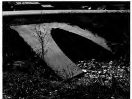
This arch pipe is sized to carry the predicted 25-year flow, but causes backwater at the 100-year flow.
