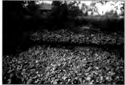
This gabion basket was undercut because of inadequate footing.
