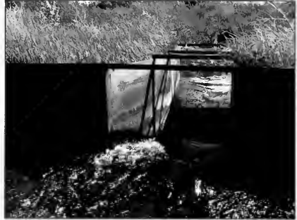
Parshall flumes cause minimal backwater, and work well in low-gradient applications.
