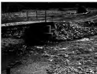
Stacked median barriers often make poor abutments. The absence of wingwalls, footings, and a 1:1 fill slope mean this bridge is likely to require additional maintenance.
