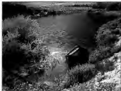
Canal checks, or outflow pipes, are commonly used on small ponds to control water elevations. Canal checks and standpipe structures do not substitute for emergency spillways.
