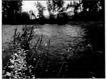
Dormant willow poles are effectively placed with a dibble on an excavator or backhoe.
