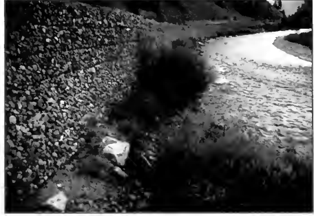
An engineered gabion wall with a rock toe prevents abrasion of wire and undercutting of the footing.
