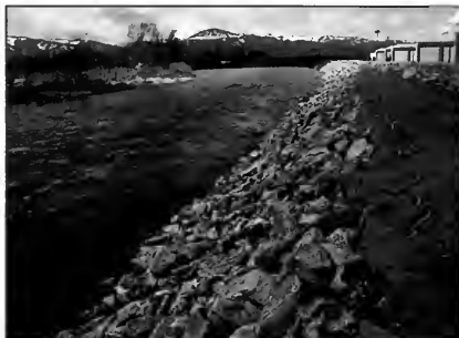
An engineered rip-rap bank provides a high degree of protection, but diminishes natural river values.
