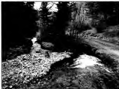
Aggradation from a failed culvert crossing has decreased channel capacity and increased flood risk to the road that has encroached on the floodplain.
