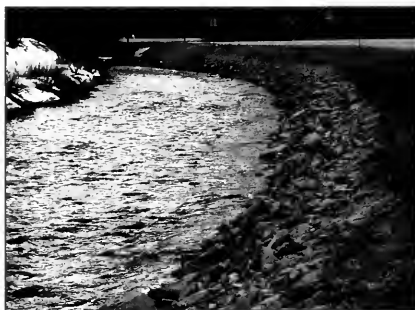
A well designed rip-rap job has 2:1 slopes and does not encroach on the river. This bank could probably have been stabilized using geotextile and vegetative methods with equal success.
