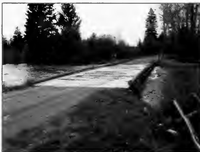
This bridge stringer is set at bankfull height. Projects should avoid this situation, which traps debris.
