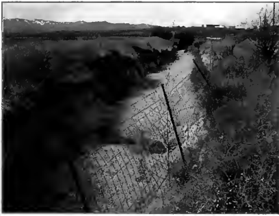
Degrading (scouring/downcutting) channels are common when streams have been straightened.
