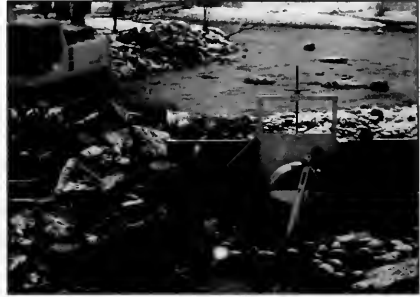
Careful design helps reduce impacts to the stream and cuts maintenance costs on irrigation diversions.
