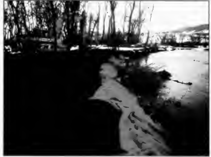
Brush layer technique is used here in combination with coconut fabric to restore the bank and enhance habitat.
