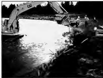
Willow fascines are being staked at the toe of the bank prior to wrapping the slope with geotextile fabric.
