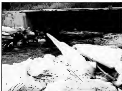
This bridge stringer was set below bankfull, and had problems with ice jams and flow capacity.
