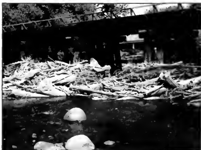
Debris jams are often associated with center piers on bridge crossings. A clear span is preferable to piers.
