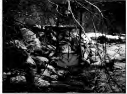
A C-10 gate generally benefits from a headwall to stabilize fill. Rock can work, but the slope leaves the gate frame exposed to ice and debris.
