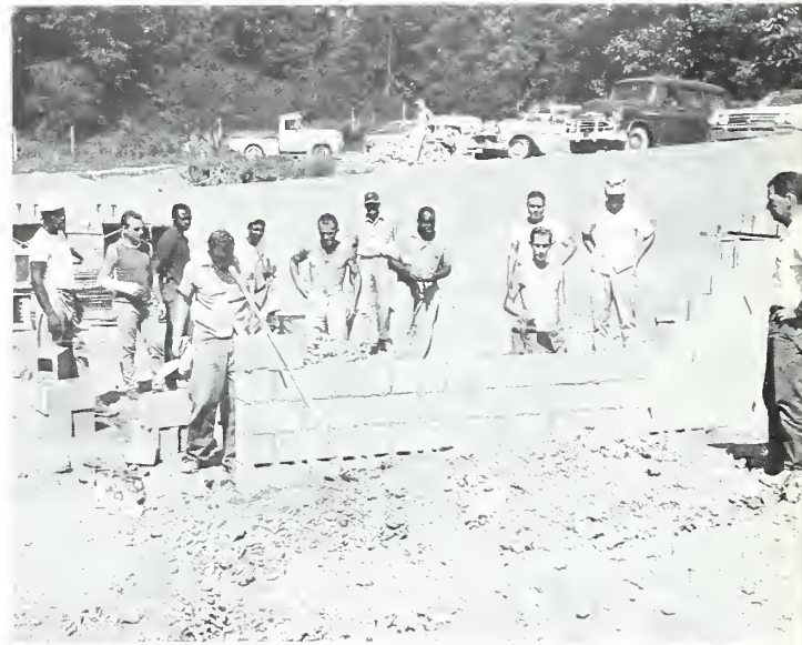
A fine example of the skills of the Brick and Block-Laying class.
