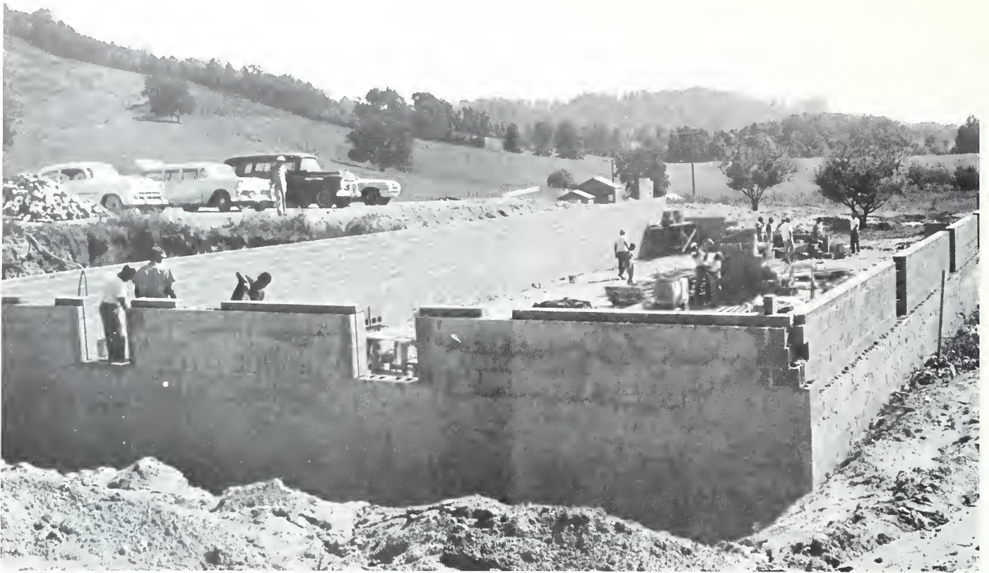
M. D. T. A. Bricklaying class constructing main building of the training grounds of the Buncombe County Fireman's Association with materials furnished by the Association.
