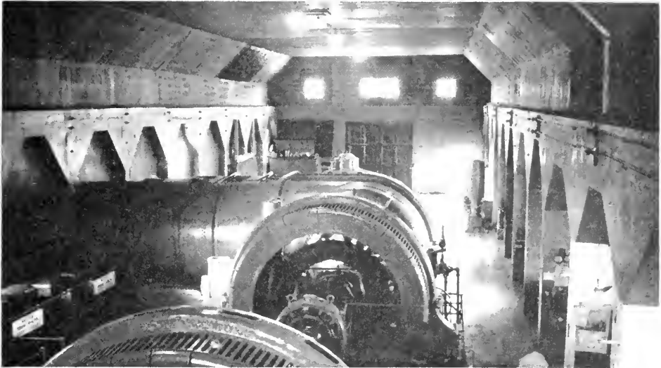
A POWER DEVELOPMENT ACQUIRED BY HYDRO Sandy Fall generating station, Mattagami river—No. 2 Unit
