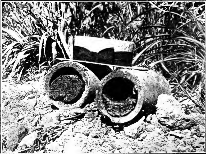
Evils of a defective siphon illustrated. The sludge has escaped into the sub-surface tiles which have been uncovered.
