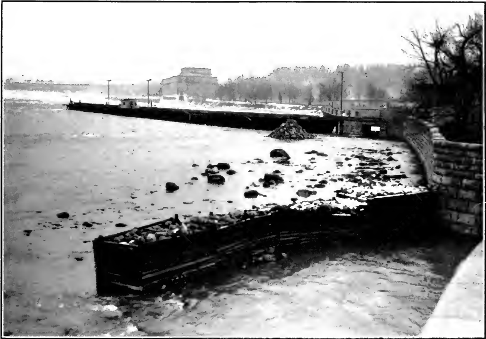
Canadian Niagara Power Co. Weir in Niagara River in the course of construction
