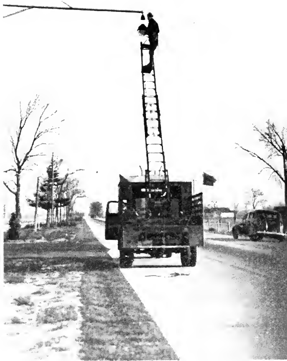
LIGHTING OF DUAL HIGHWAY, TORONTO TO BURLINGTON Truck with extension ladder for installation and maintenance
