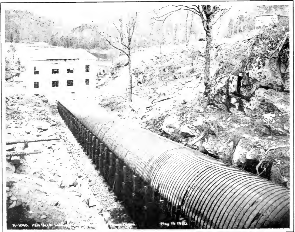
High Falls—Looking down Penstock to Power House.
