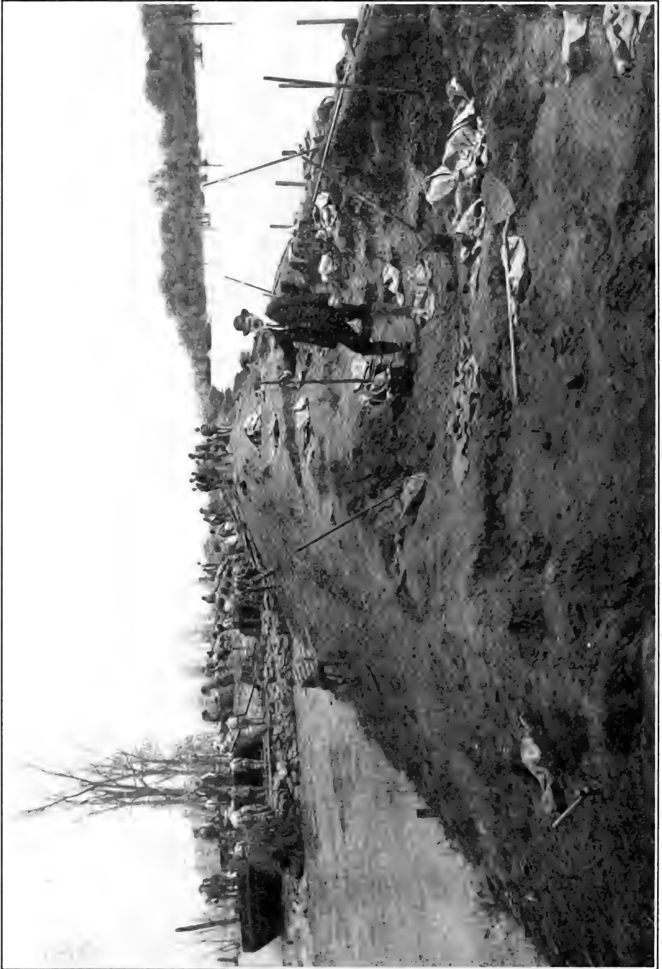
Strengthening the Levees in Preparation for the Coming of a Flood. Lagrange, Mississippi, 1903
