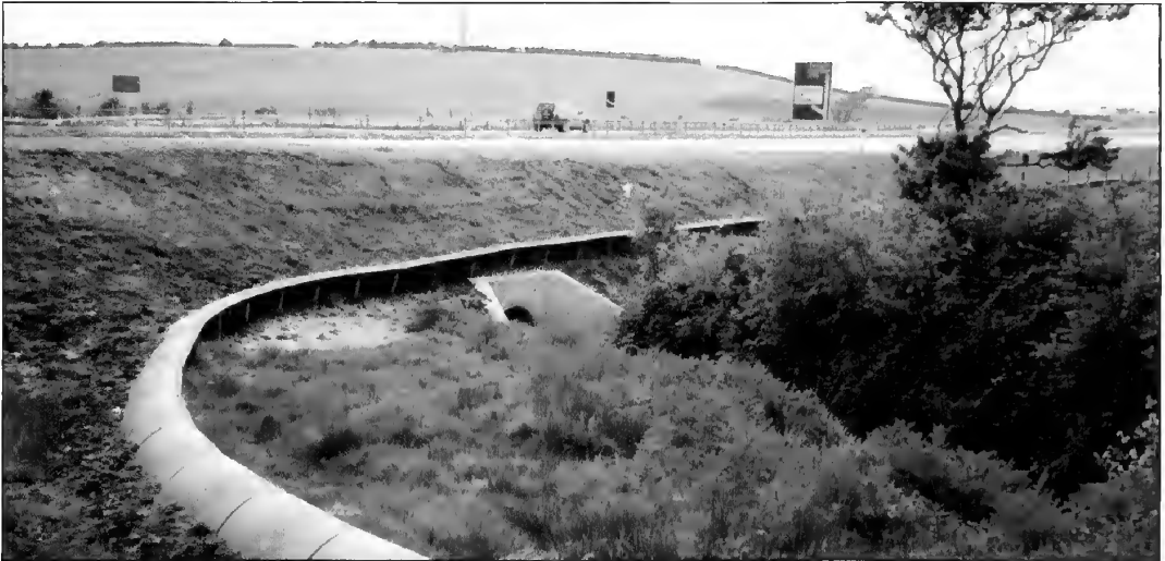
A combination of barricade and culvert provides safe passage for wildlife.
