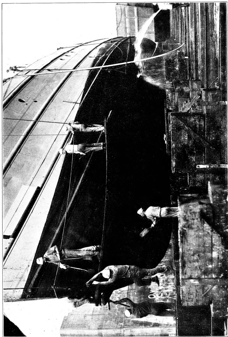
FIG. 1.—Process of cleaning the hull of a ship after dry-docking. The U. S. Ouel at the Norfolk Navy Yard, June 6, 1925
