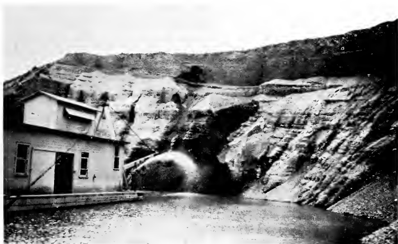
Figure 14 Hydraulic jet loosening a 50-foot face. This lessens the danger from sliding and also feeds material to the pump
