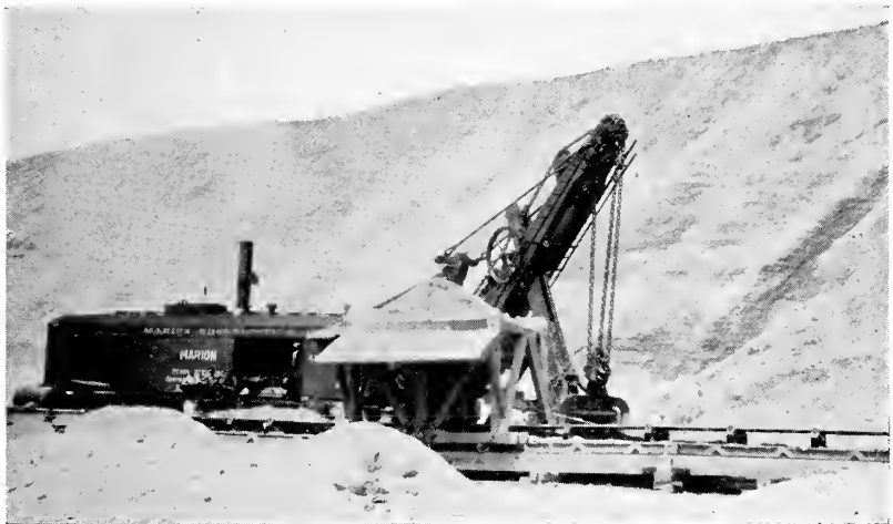
Figure 11 An efficient method of excavating and conveying material. For a detailed description see page 70
