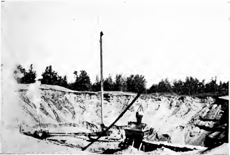
Figure 10 A stiff-legged derrick with a clamshell bucket dumping into a hopper protected by a grizzly
