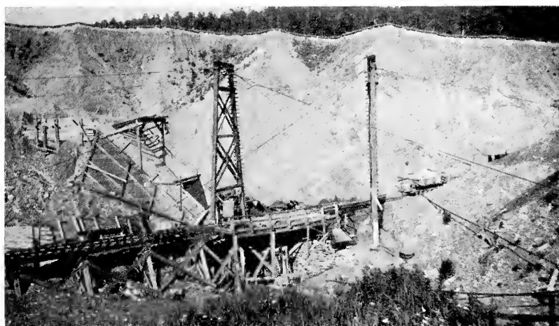
Figure 28 Excavating being carried on simultaneously by a steam shovel dumping into pit cars and also by a drag line
