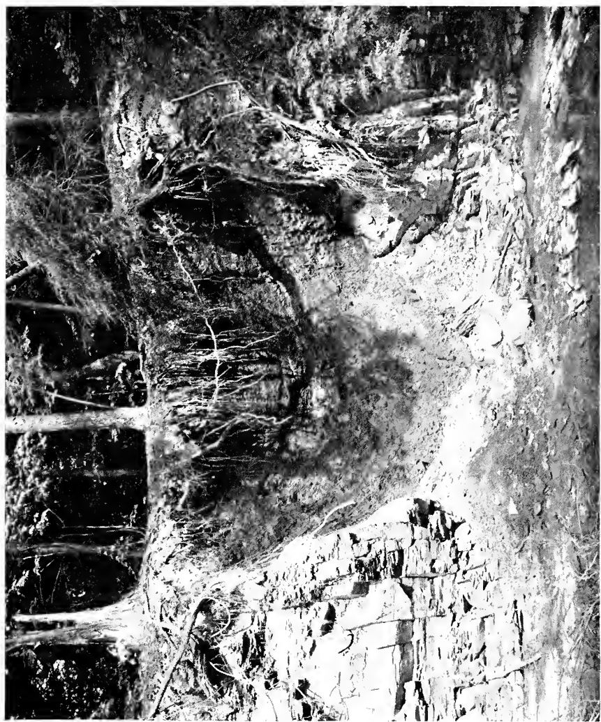
Figure 24 Filled gorge cut into Genesee shale at Bellona, N. Y., before clearing and excavating the site (June 6, 1929)
