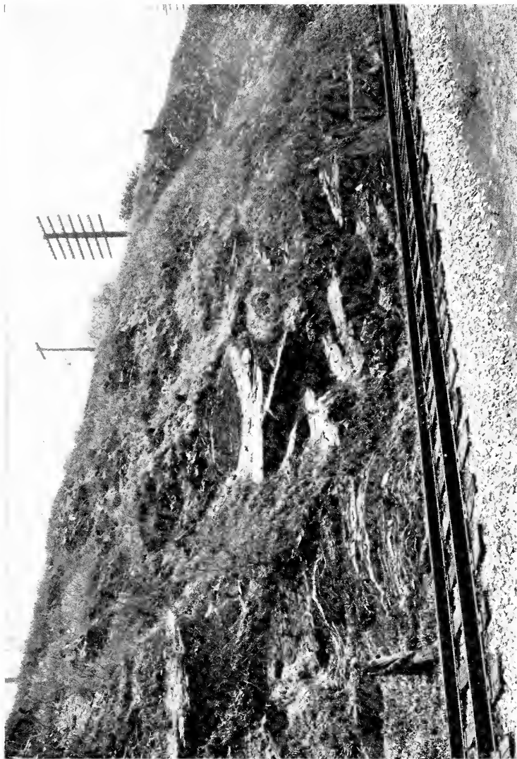
Figure 19 Deepkill shale at the south end of the cut along the New York Central railroad tracks, south of the Stuyvesant railroad station. View southeast. Note the characteristic calicheous bands near the figure. (Photograph by E. J. Stein)
