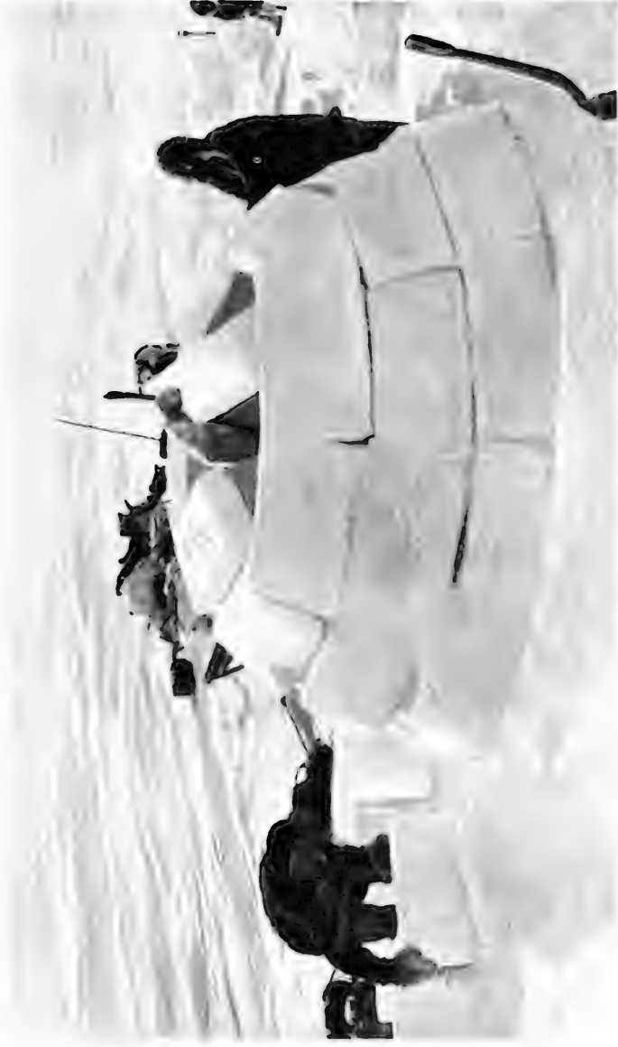
Building the snow house. From "The Friendly Arctic." Courtesy of Mr. Vilhjalmur Stefansson
