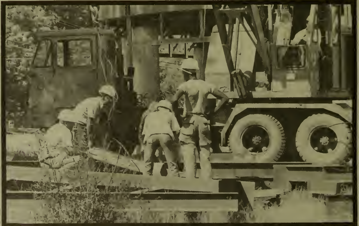
Workmen struggle with pieces of steel framing as construction gets underway on our new classroom building — from the ground up.
