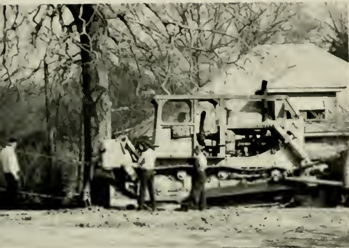
This is the tractor attached to the cables, waiting to pull the tower down.
