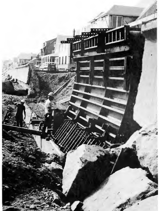
Because they reflect the force of storm waves back onto the beach, sea walls tend to undermine themselves and collapse. Here a section of wall in Marshfield, Mass., is replaced after its destruction in a 1978 storm. (Photo by Jeff Benoit, Mass. Coastal Zone Management)
