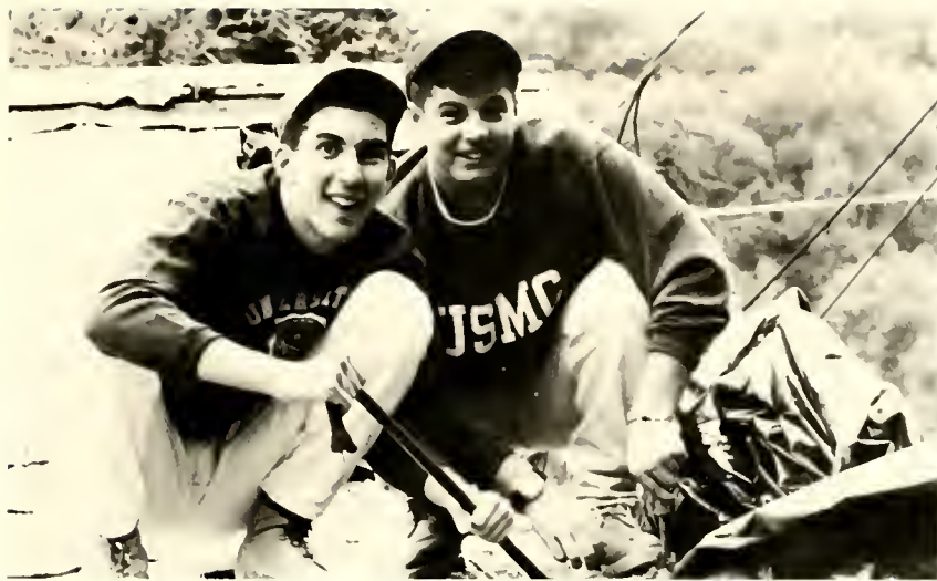
Greg Humphries (left) and Mike Hernandez are patching up a tin roof on a home in Avery County as part of their Alpha 101 service project.
