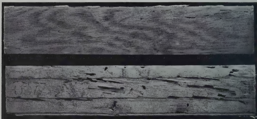
Fig. 8.—Oak flooring damaged by termites. The top view shows the varnished surface of the flooring. The lower view shows the concealed damage to the same board done by termites. This illustrates the difficulty of detecting termite damage on exposed surfaces. Often entire boards are destroyed except for the very thin exterior layer of wood.
