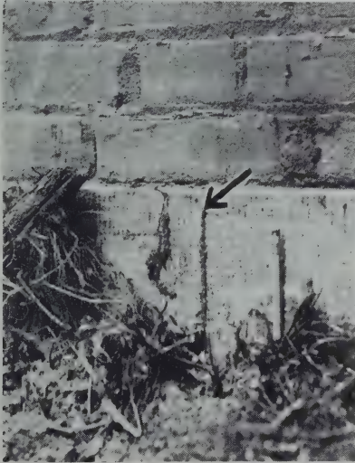
Fig. 6.—Termite tube built up on the outside of the concrete foundation of a house. This tube is small and rather difficult to detect. The foundation must be carefully examined to locate such inconspicuous tubes.
