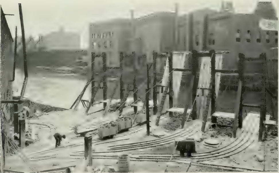
FIG. 9. TRACKS AND MOVABLE PLATFORMS. For dumping the excavated clay into scows in the river.
