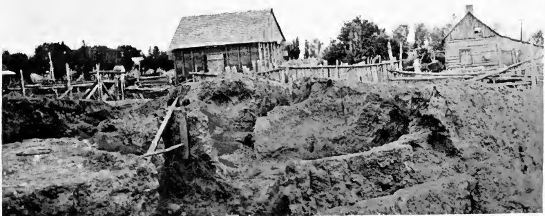
Kiva I from the north wall of Room 2, shown at the lower right; Fireplace B at the left of the braces which support the east wall of the ceremonial room.
