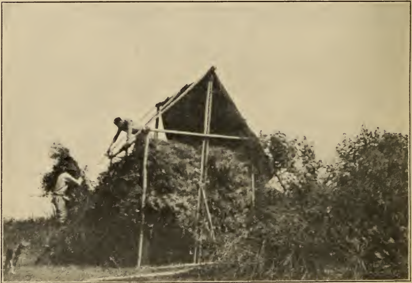
FIG. 2.—PERMANENT CURING SHED 8 BY 16 FEET. BUILT OF BAMBOO POLES WITH ELEVATED PLATFORM. CAPACITY ABOUT 2 TONS CURED PRODUCT. COST ABOUT $5.
