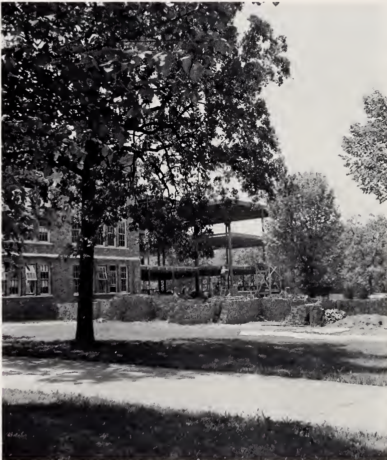
The new wing, constructed during the summer and fall of 1962, added 12 classrooms to the facilities of Central High School.
