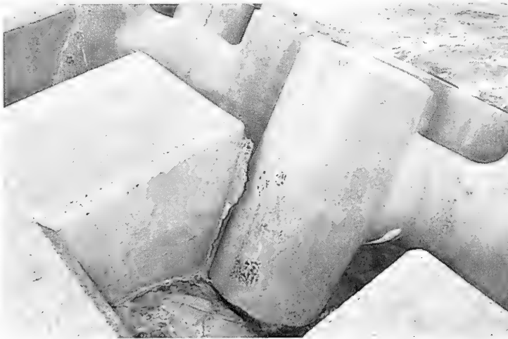
Figure 11. Separation between tribar and rib cap
