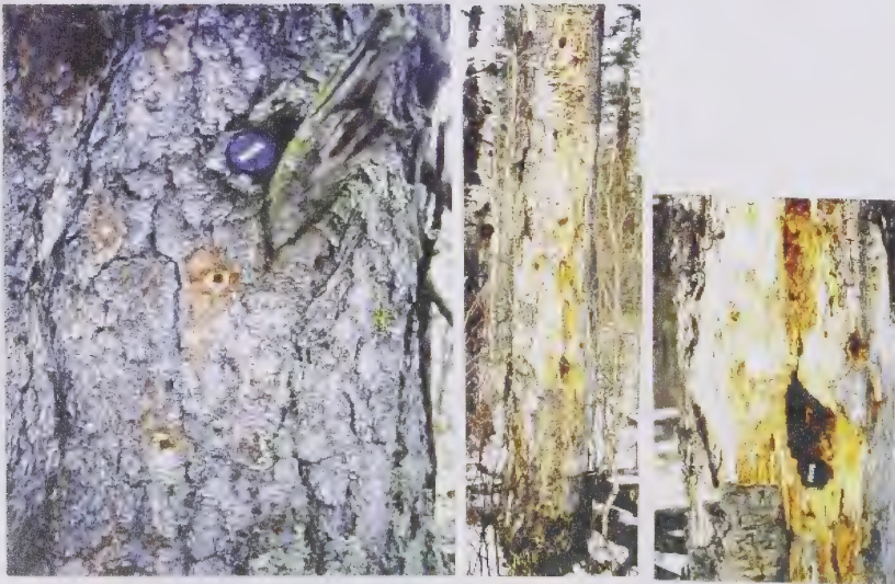
FIGURE 4.16 EXCAVATIONS BY WOODPECKERS
