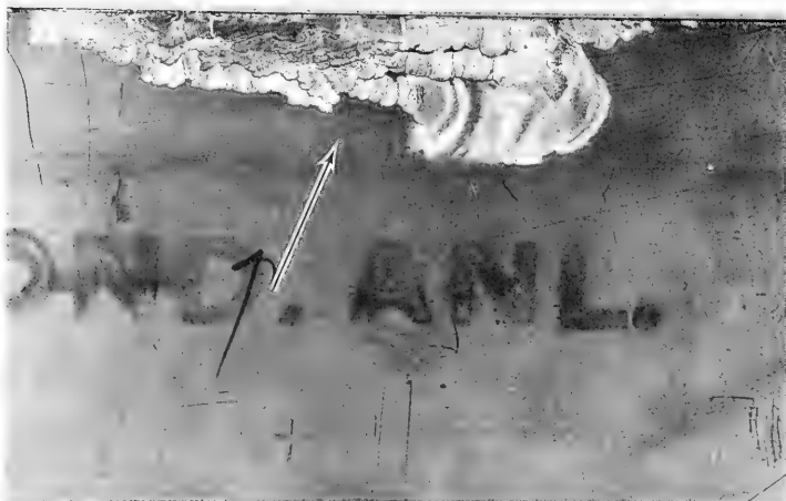
Figure 11. Close-up of a stainless steel panel, showing crevice corrosion at the edge. The corrosion occurred underneath the TFE film where seawater had leaked inside through small ruptures.
