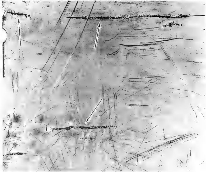
Figure 15. Close-up of stainless steel control panel showing elongated corrosion (tunnel pits). Tunnel pits were not found on protected panels.
