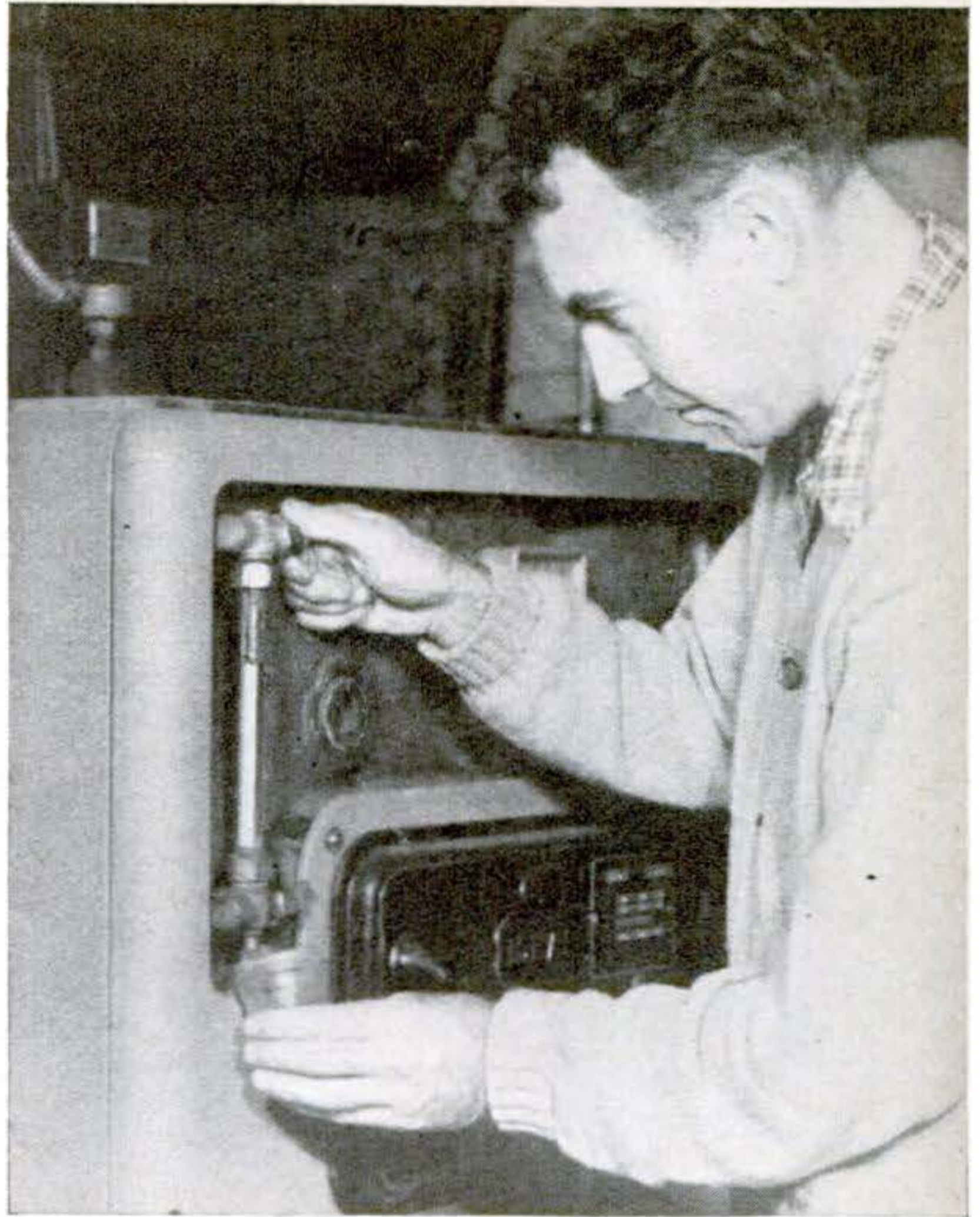
WATER GAUGES can be cleaned when the furnace is in operation with an acid solution drawn up by vacuum action
