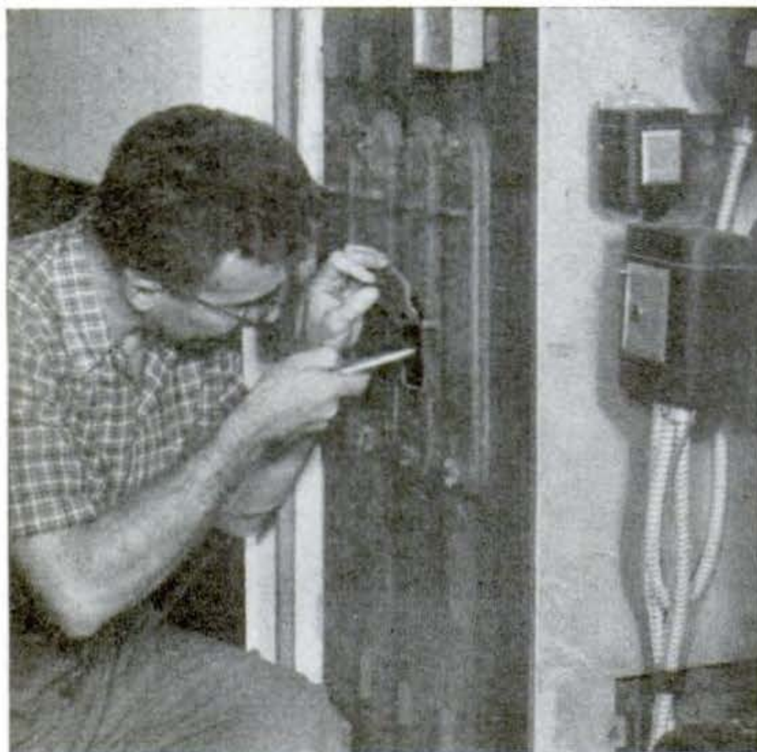
CRACKS in some boiler sections can be seen through a peephole with the help of a flashlight
