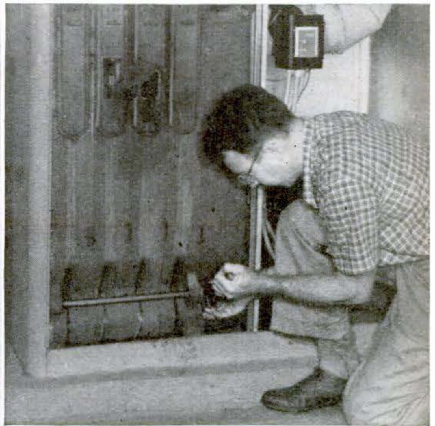
LEAKY JOINTS are stopped by tightening the tie-rod nuts and then turning them back again
