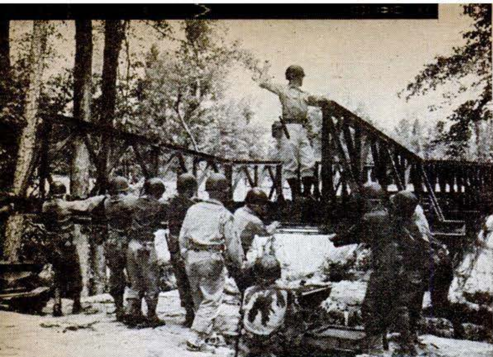
On the far bank, another pair of rollers has been set up and a part of the crew is ready to receive the launching nose as it inches over. Standing on the nose, the officer in charge directs the ticklish job
