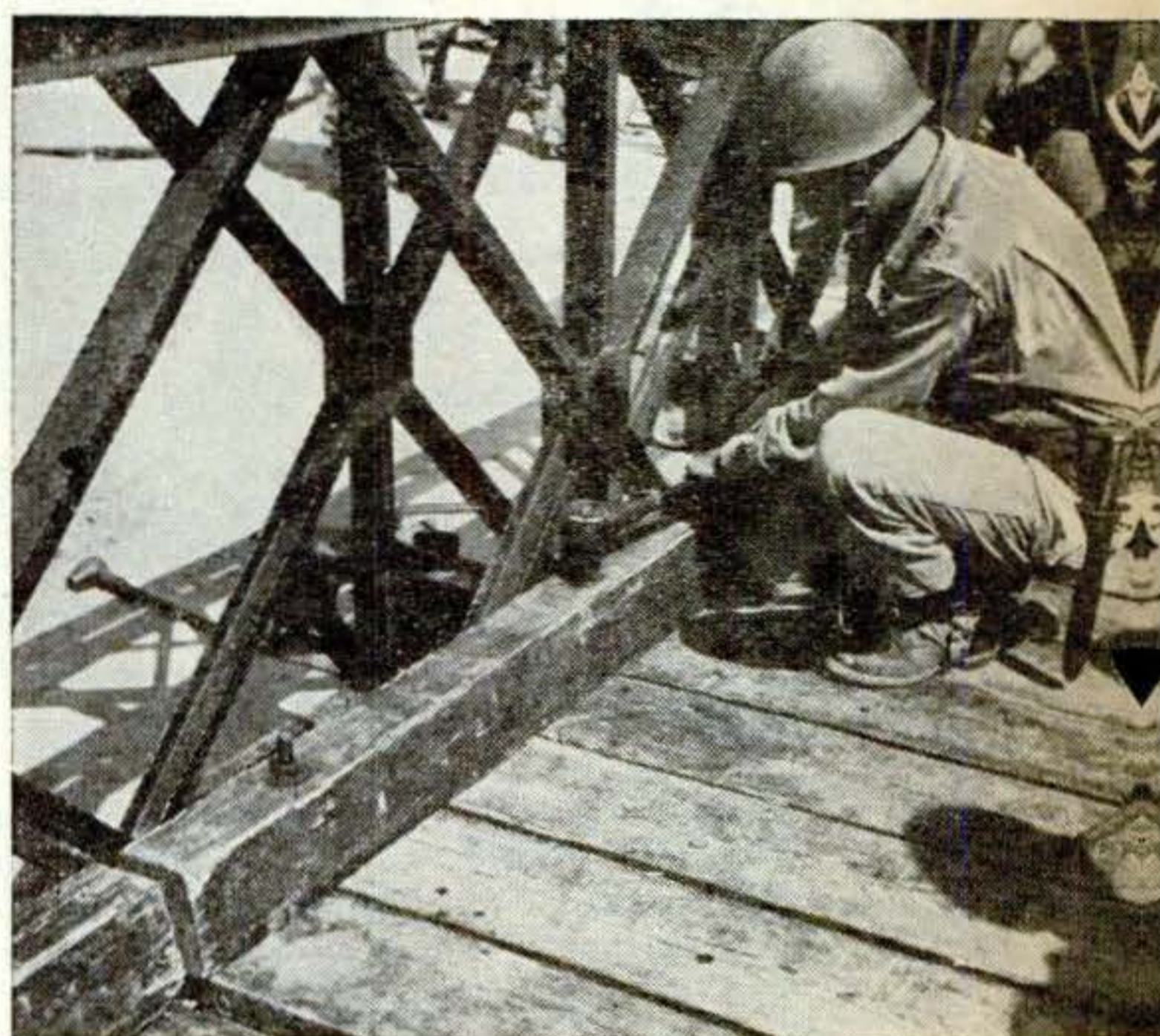
One curbing plank covers the ends of 13 floor planks. Four bolts, which go through the curb planks and engage with the stringers, hold down the ends of all 13 planks. This completes the flooring of the section
