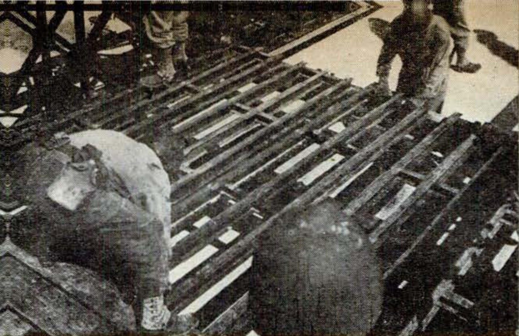
These men are laying the stringer units, which fit neatly into lugs on the crossbeams and need no bolting. All parts of the Bailey bridge are designed to go together with a minimum of labor and to require the smallest possible number of tools and fittings
