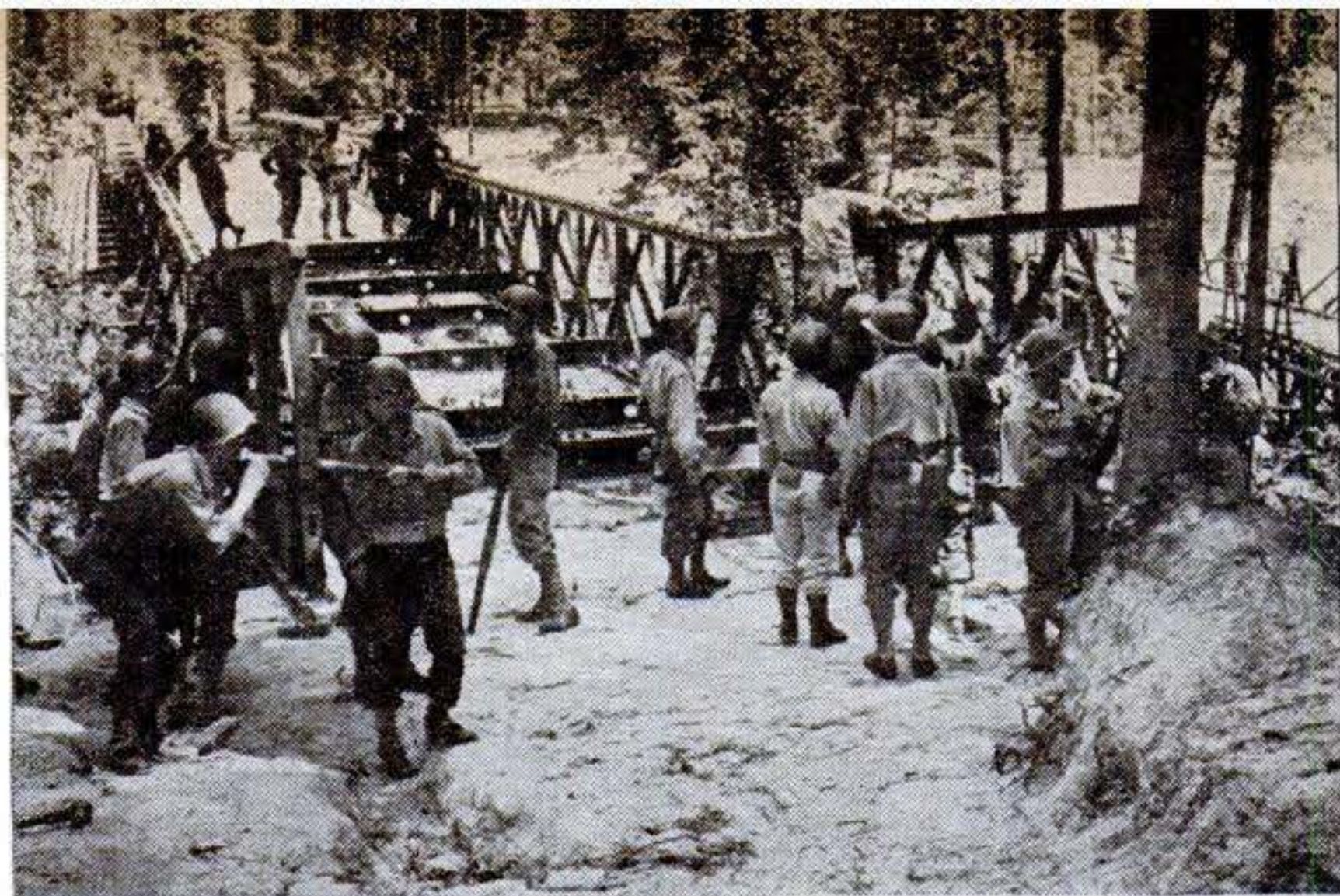
The bridge now rests on rollers at both ends. As the additional sections are added on the opposite side, it is pushed over and the launching nose is taken off, part by part. A bulldozer often helps with the pushing
