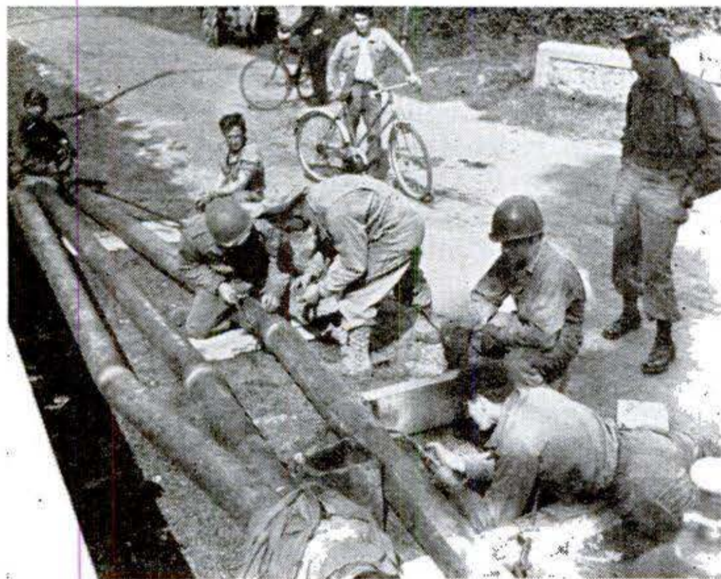
Below, sections of the pipe-line system laid by Army engineers to carry water and gasoline across France are welded together with portable outfits.
