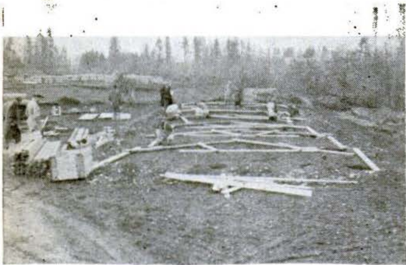
3 Parts for the framework are laid out on the ground. Wood is soft or yellow pine, while the covering material is sheet or corrugated steel.
