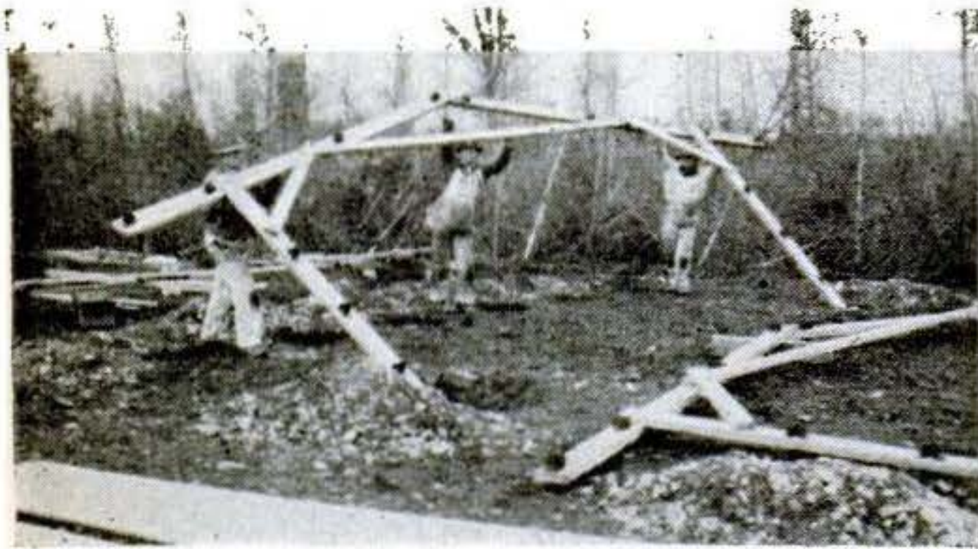
5 House-raising begins with one of the end sections as the posts are set in shallow holes. It is not necessary to level the site perfectly.
