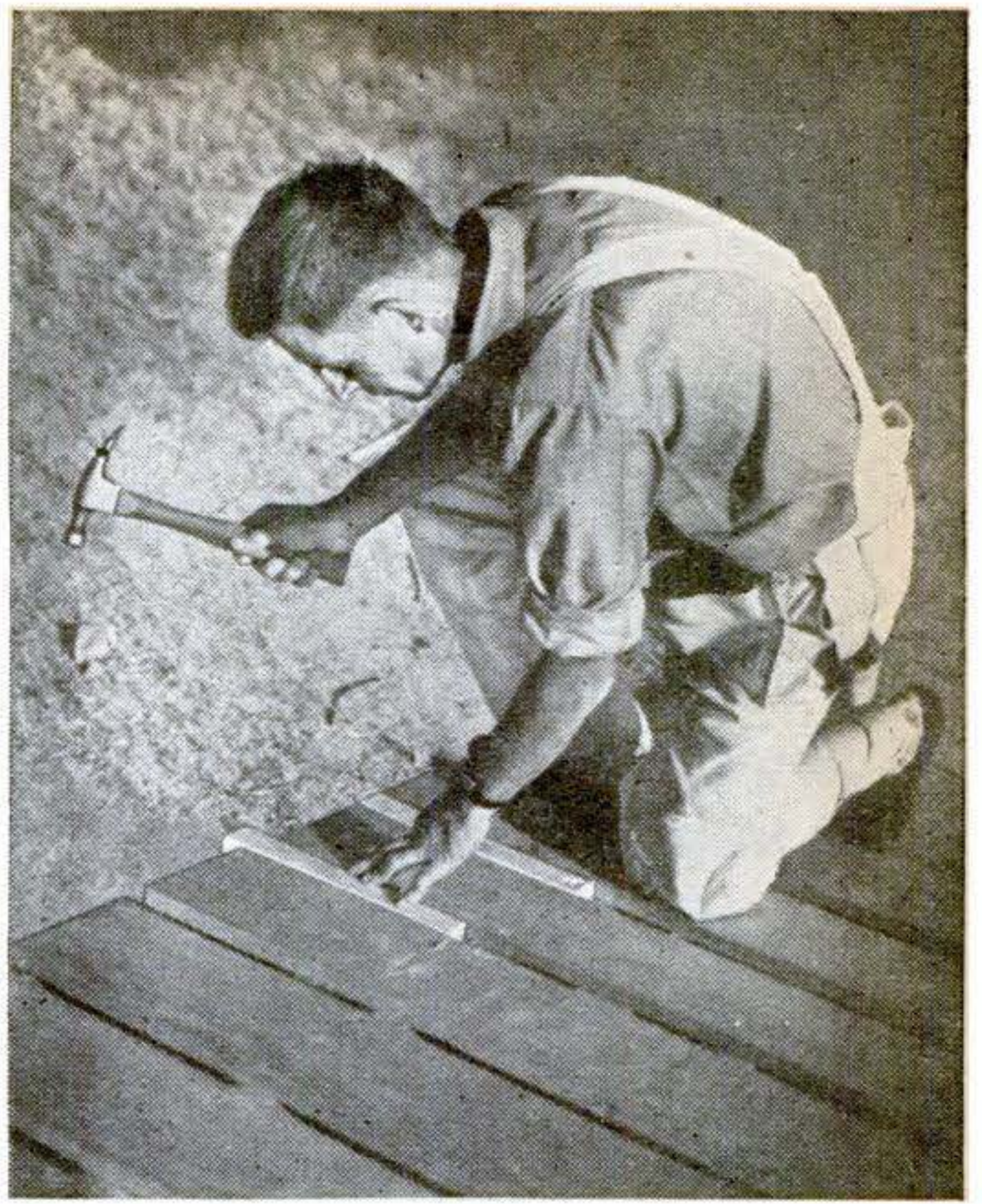
Short lengths of filler strips may be nailed in between the sheathing from the barge boards to the first rafters if a rustic effect with shingles showing through is not desired.
