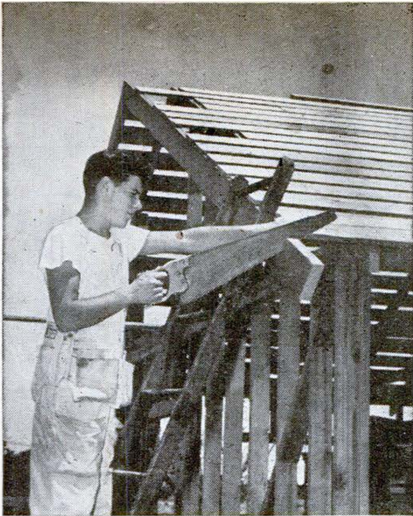
When both the barge boards have been permanently nailed in place, plumb a line at the ends and saw them off vertically to length. They are held to the roof simply by nails through the sheathing.
