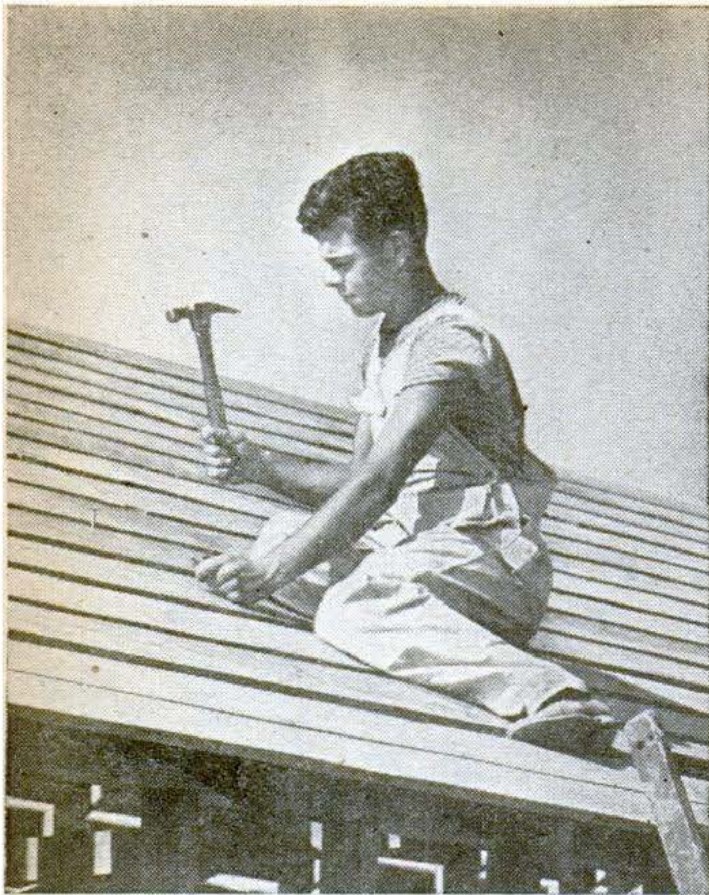
Space and tack sheathing in place for an entire side, and then nail it permanently. Nail along the length of one rafter at a time. The sheathing is laid with the rough side up.
