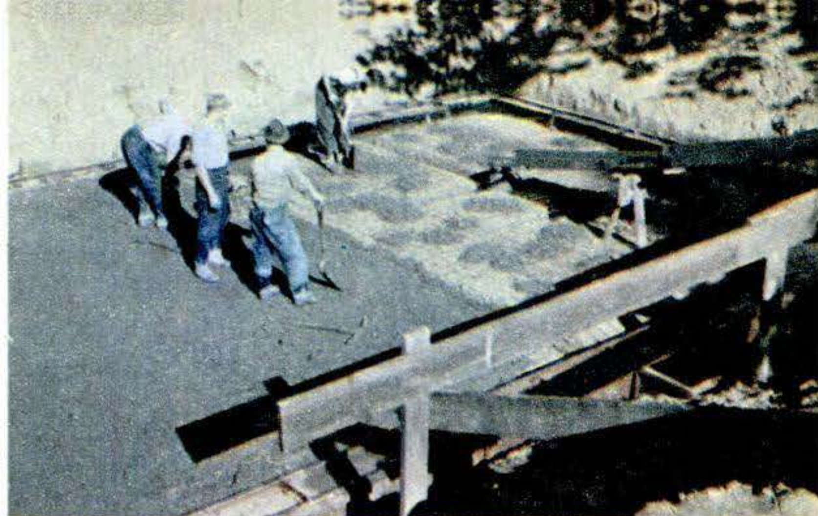
Spreading concrete over metal reinforcing of 4 1/2-inch floor of cellar, strong enough to support rockers. Cellar floor takes four truckloads of six cubic yards of concrete each. Bolts are set into floor for the control tackle.
