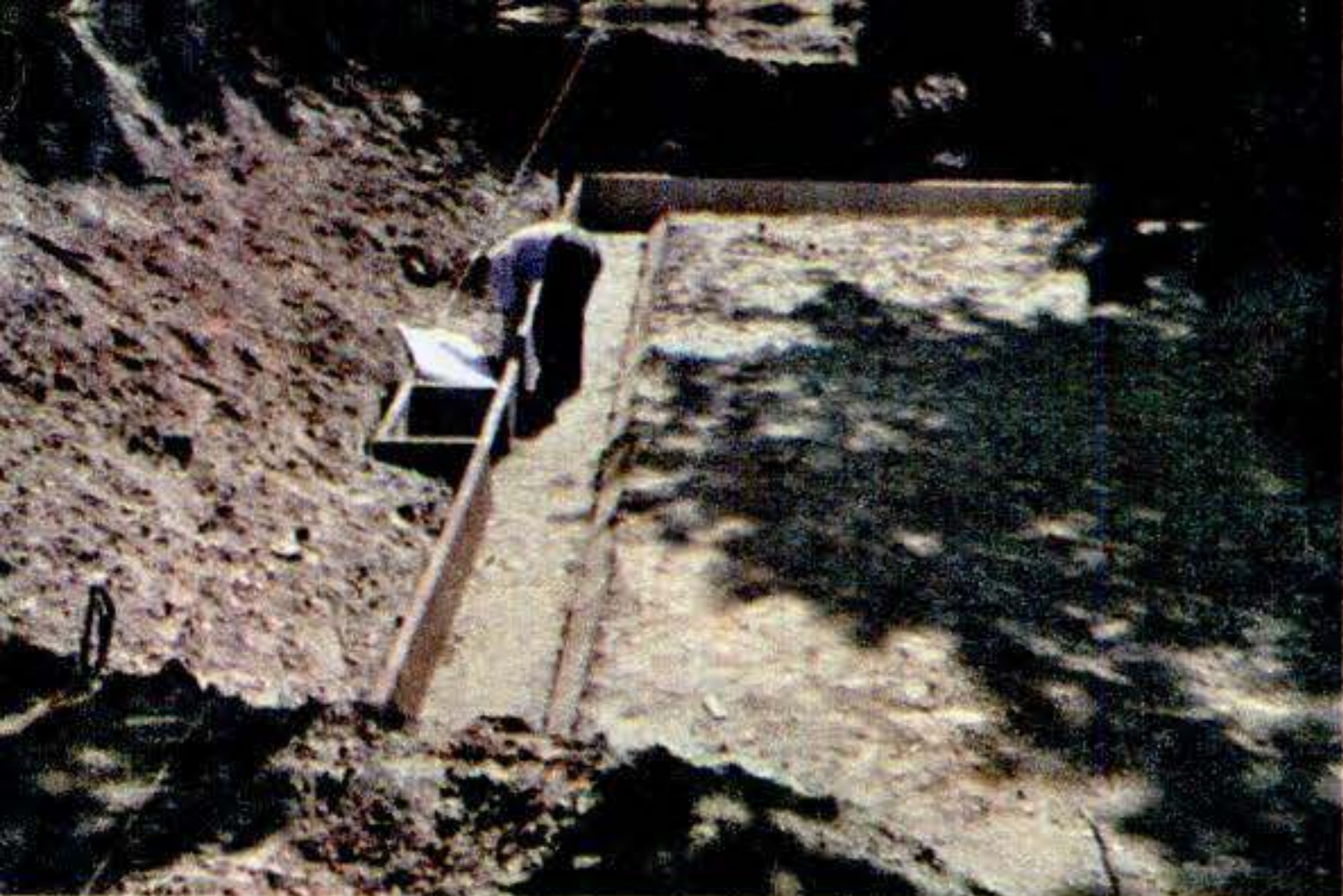
Setting up forms for the footing and cellar floor. Footing has trough slightly wider than wall, set with metal shims. When wall's foot rocks into the trough, shims support it so that a narrow opening is left between wall and footing.
