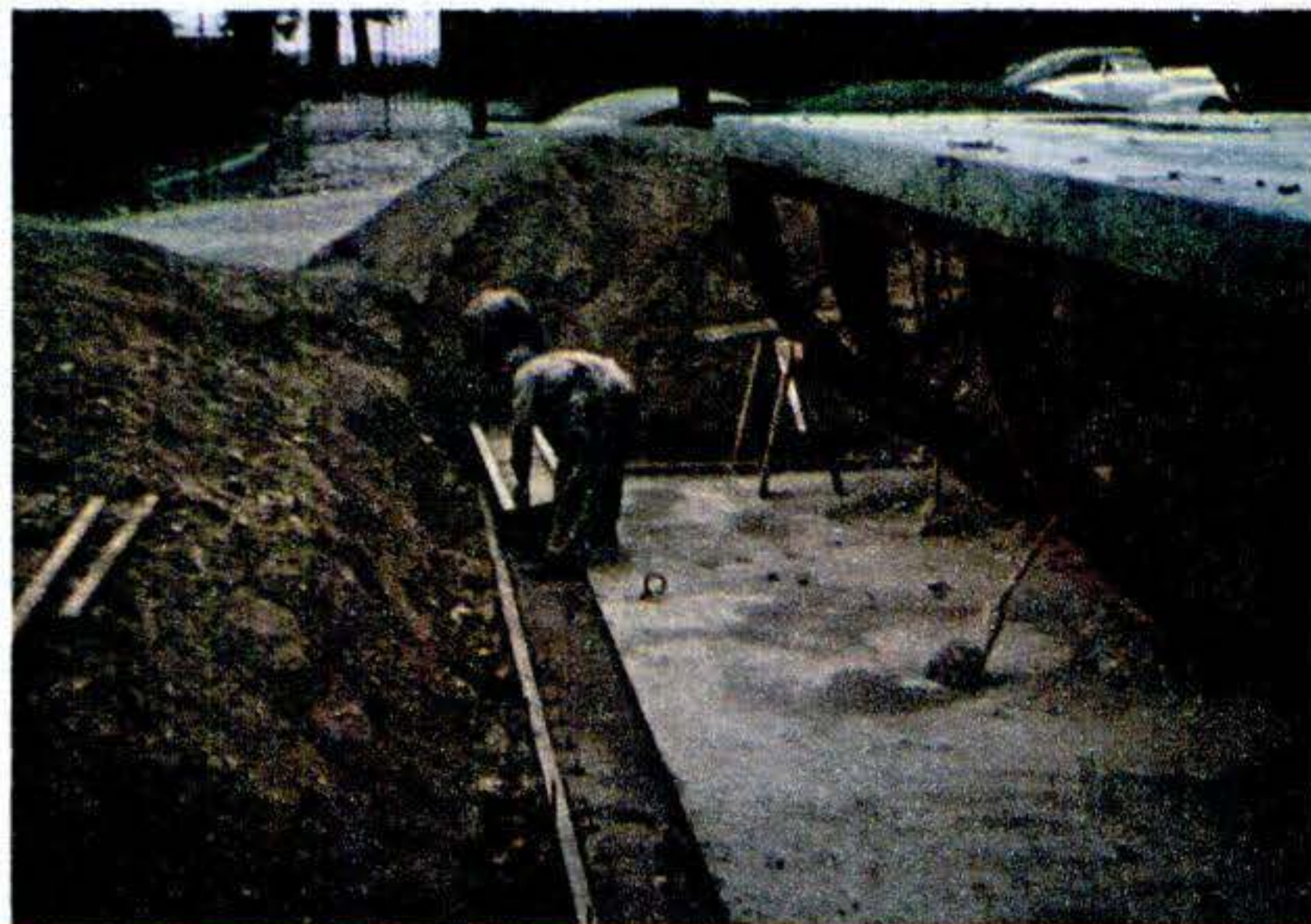
During 48-hour curing of 48,000-pound wall, workmen prepare footings. Space between wall and footing will be filled with caulking, covered with cement. Bolts to tie in floors and roof have already been put in molds so that they are set in walls.
