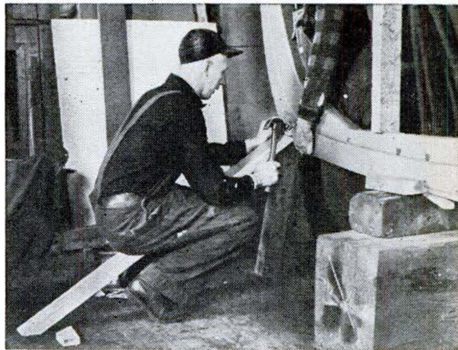
Additional braces are forced in below the first pair. Diagonals must be beveled to fit the keel just below the rabbet line and to fit solidly on the floor.
