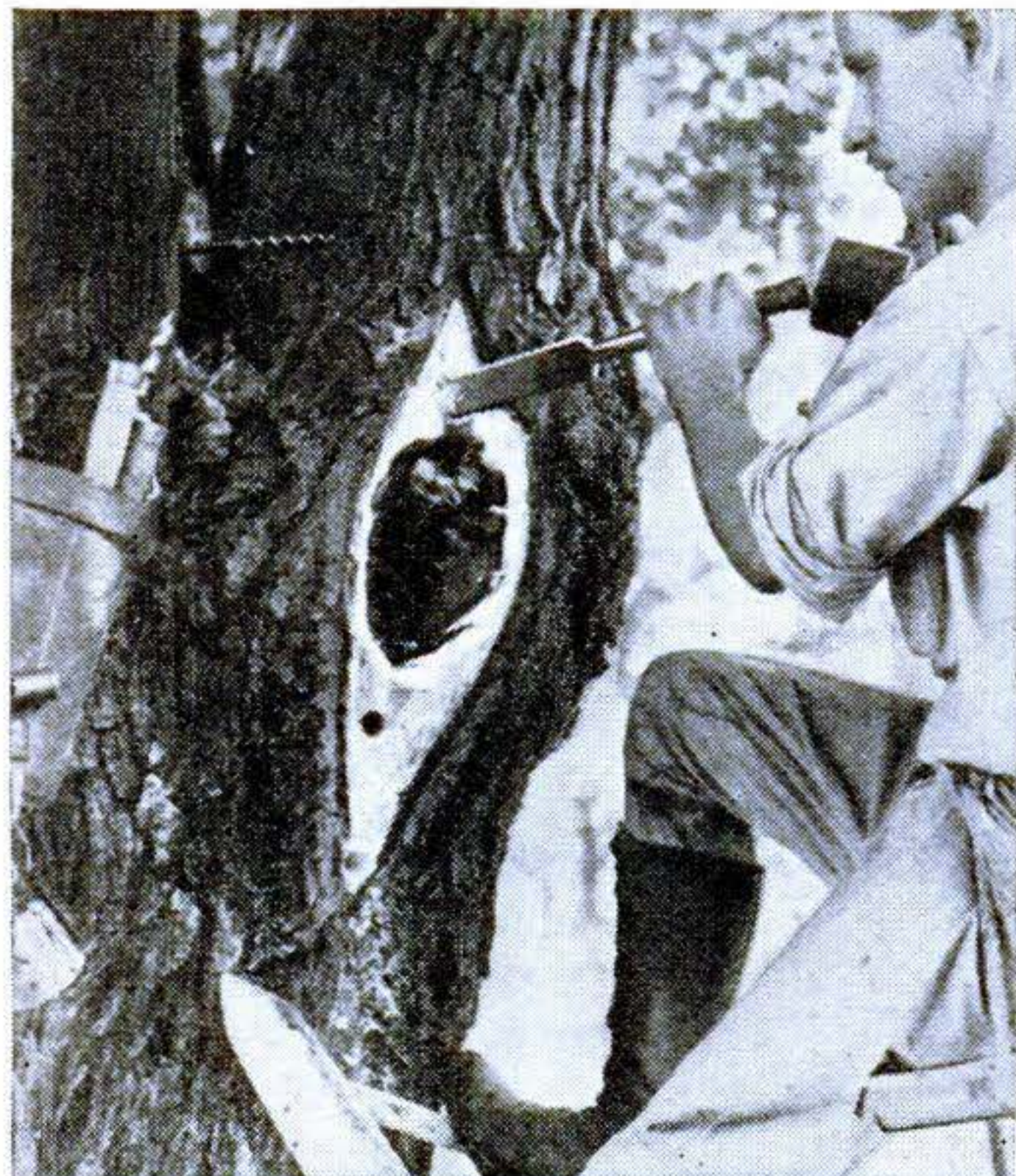
Excavation is done with a mallet and sharp chisel. Rotting matter is removed down to clean wood, and chips are cleared out so air pockets won't form.
