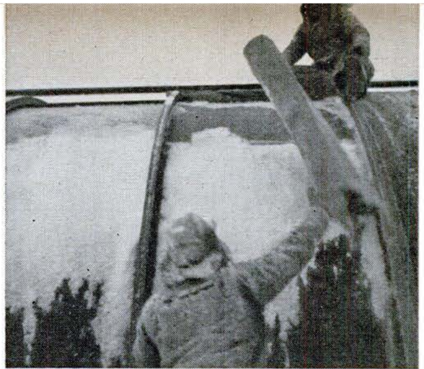
It took 600 man-hours to erect this Quonset hut. Although very warm, the Quonset is not practical on deep snow because of the difficulty in obtaining support for the foundation.
