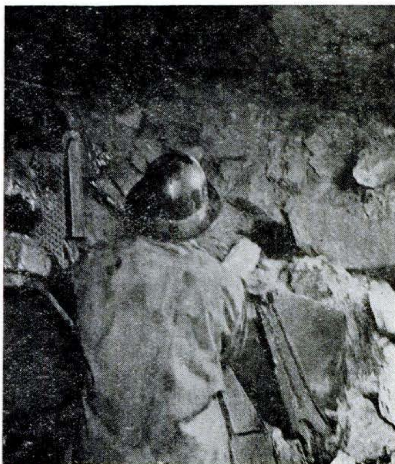
Mucking machine attacks the pile of rock thrown down by the blast. PSM's cover gives another view of the machine in action.
