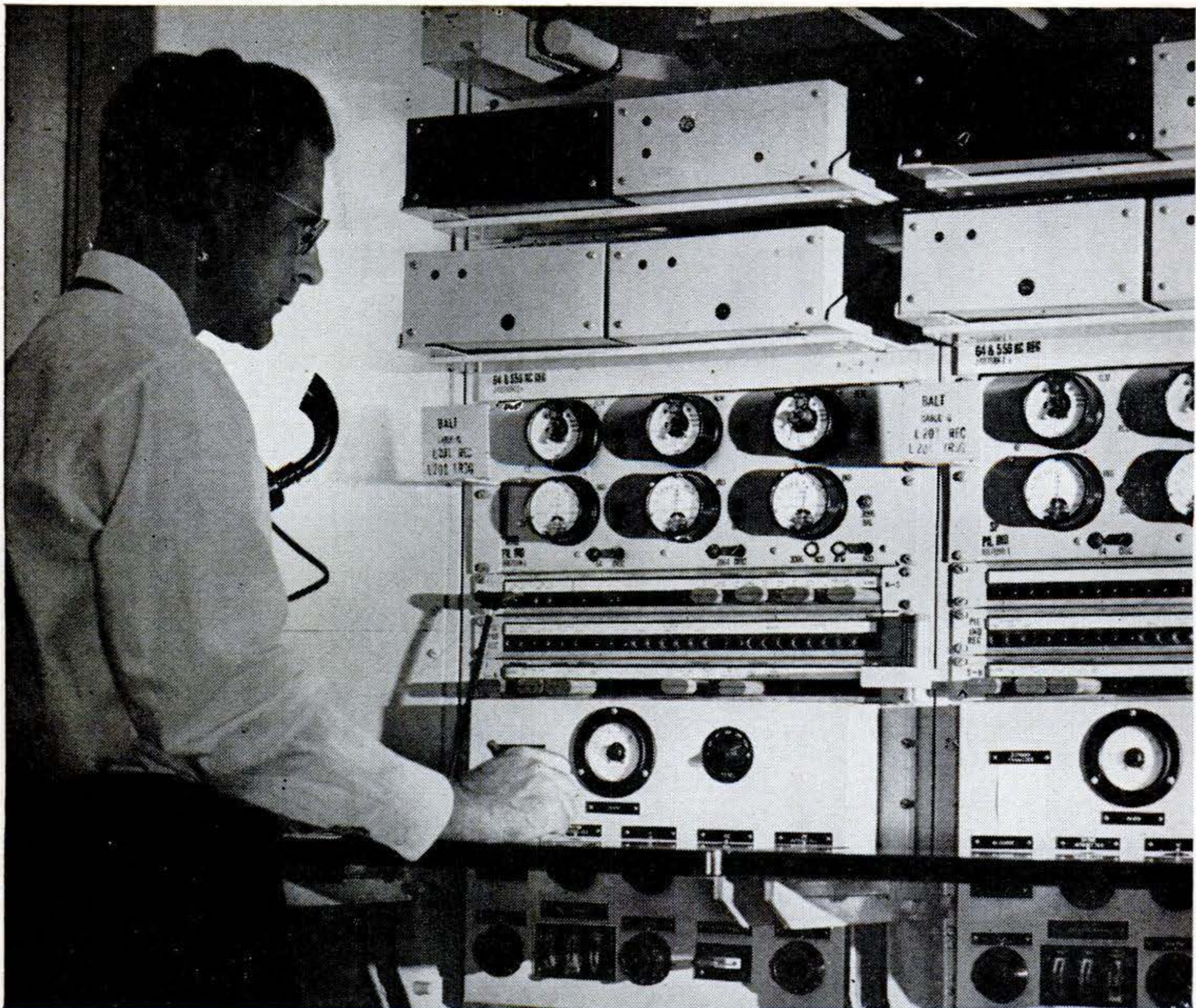
At Philadelphia, a testboard man answers as an electronic watchman calls attention to conditions on one of the coaxial systems to Baltimore and Washington.
