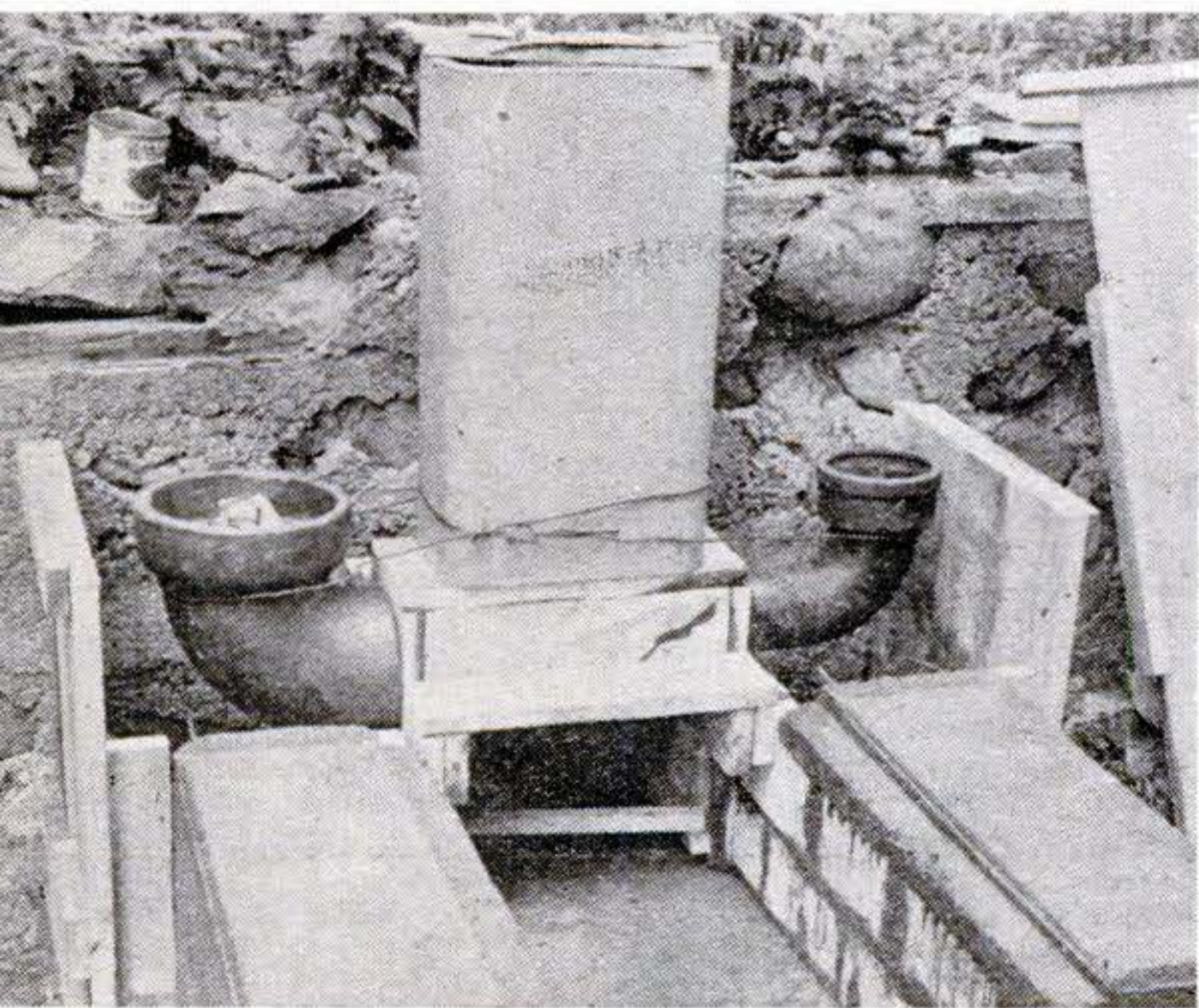
Elbows of two sizes are used for the cooking holes. Support these with wires and blocks.
