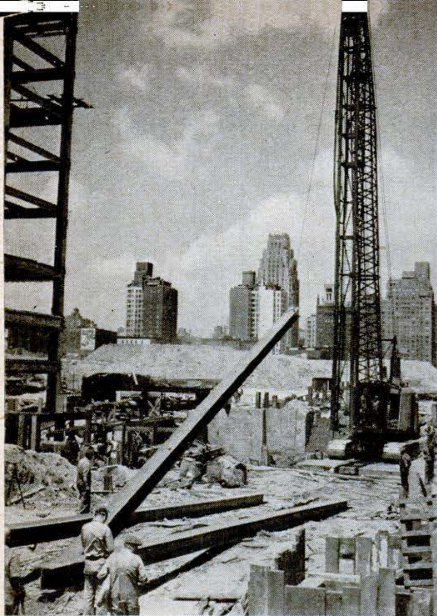
1. After big mobile pile driver has been maneuvered into place on endless tracks, cable is attached to long steel pile, and rig swings it aloft, to stand on end for driving to bedrock.
