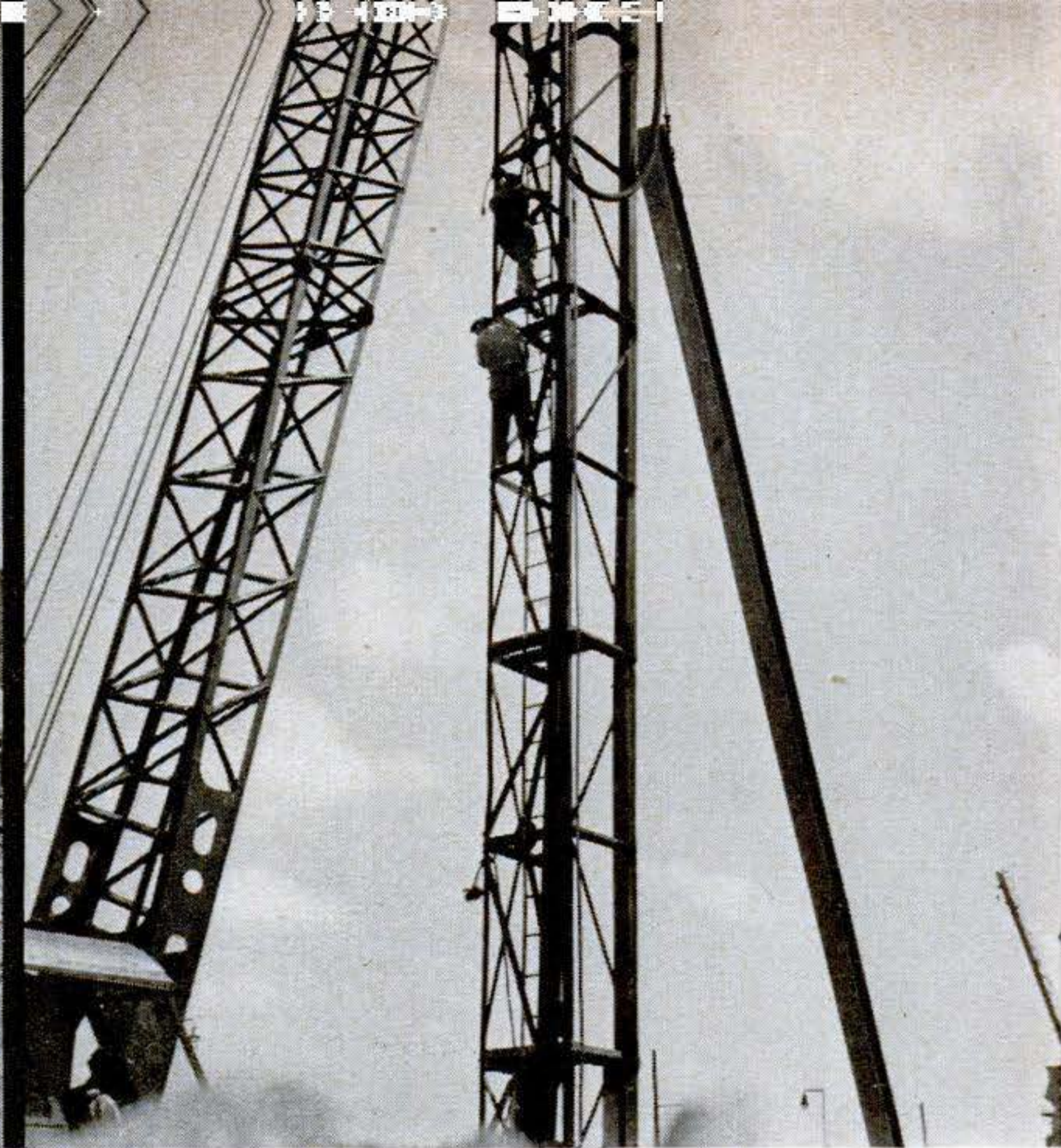
2. Men scrambling up rig, to help guide pile, give idea of its comparative size. But even this big pile driver is far from largest of type, giants that have driven piles 194 feet in length.
