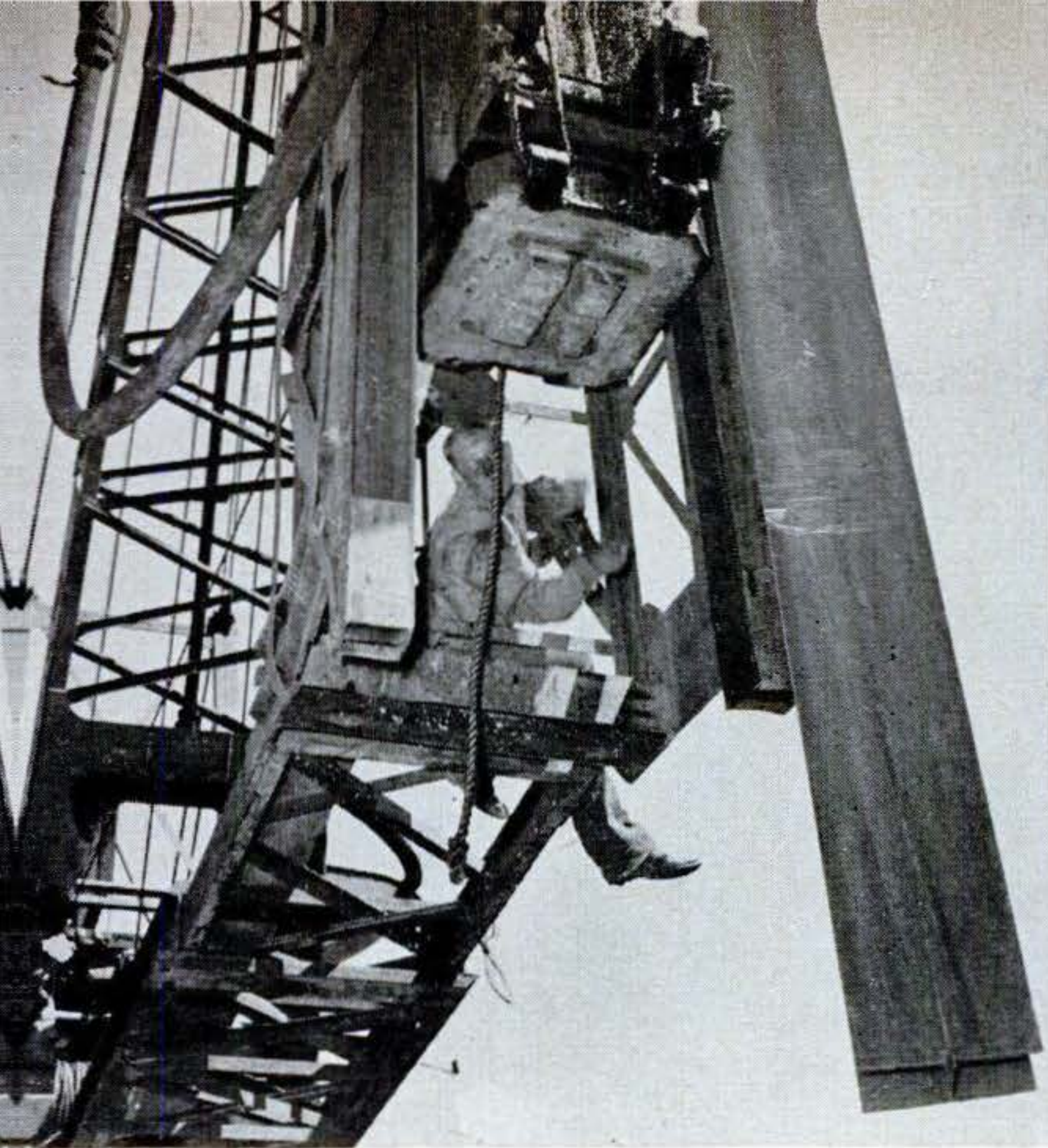
3. Worker drops rock to check position of rig over right spot. Seen just above him, anvil of steam hammer is notched to fit and engage H-shaped end of pile that hammer will drive.
