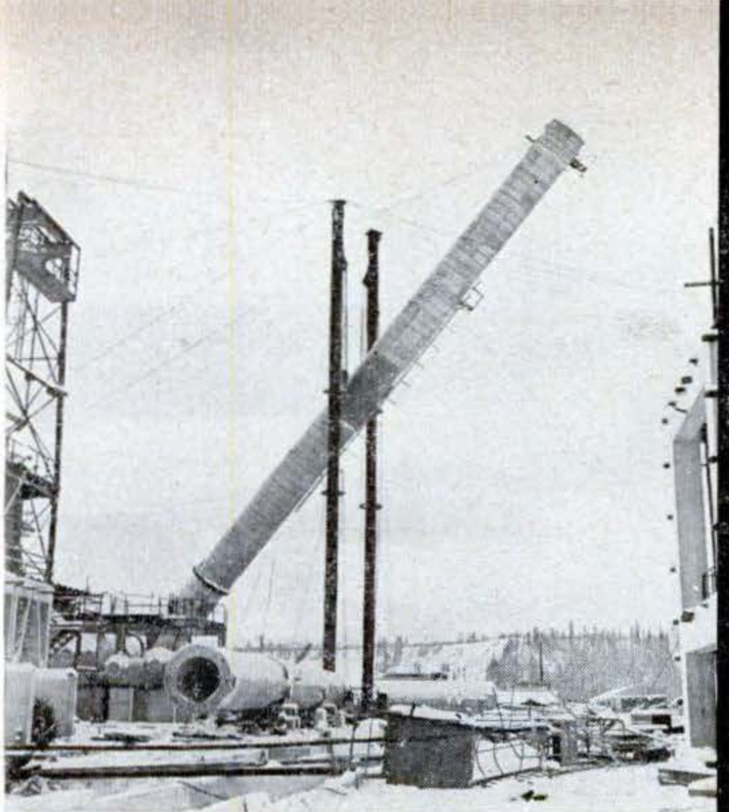
2 One of major dismantling jobs was lowering giant 146-foot refinery tower intact. Superstructure had been removed previously.
