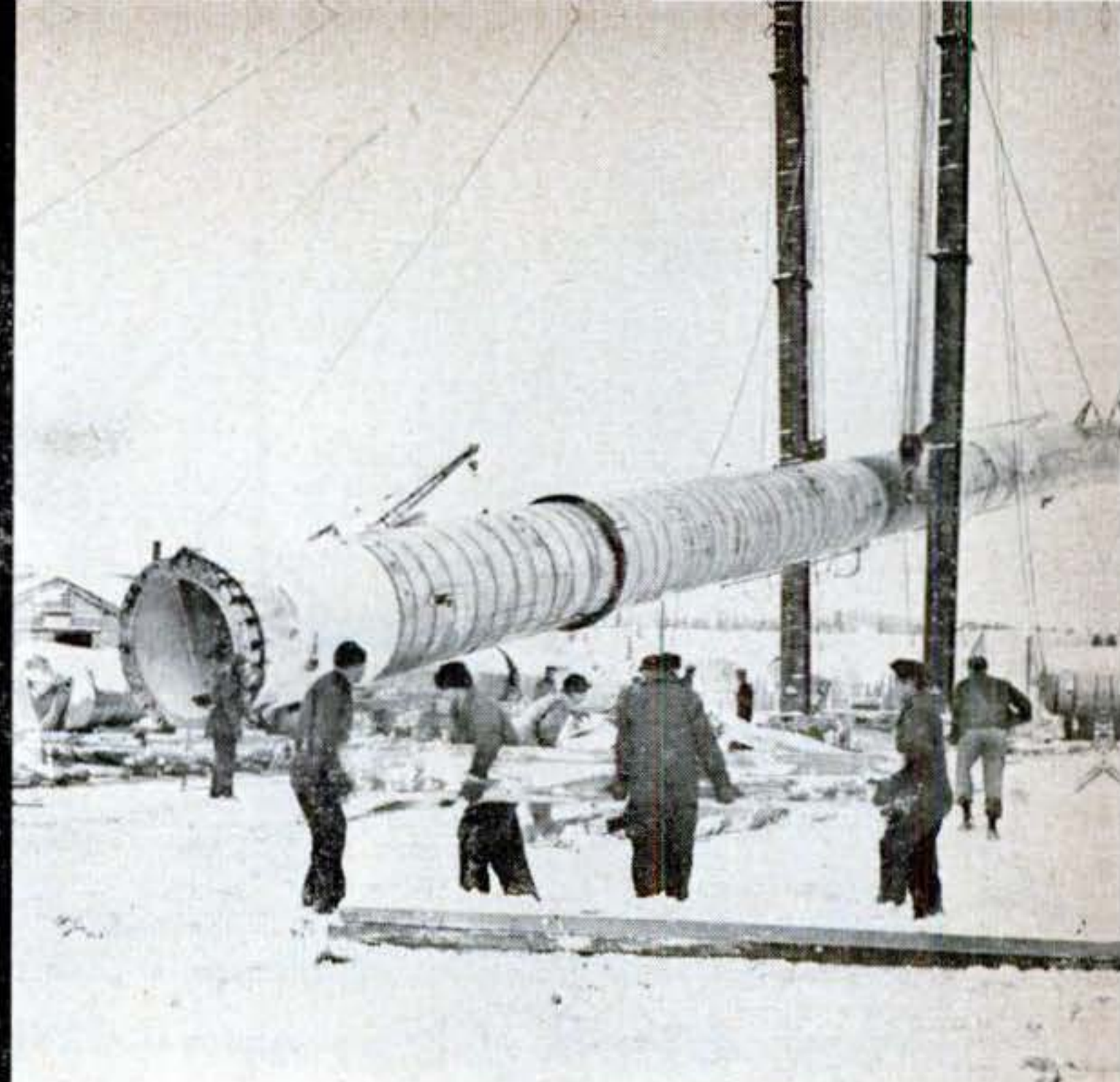
3 As the tower, held between steel rigging poles, nears the horizontal, workmen build up timber trestles to support "can" on ground.
