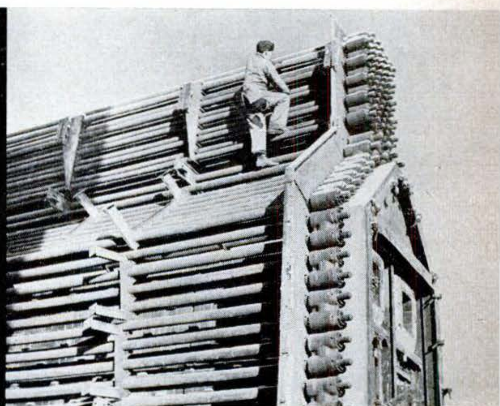
5 This log-cabin-like structure is a furnace being dismantled. Workman at top is one of many Yukon Indians engaged on the project.
