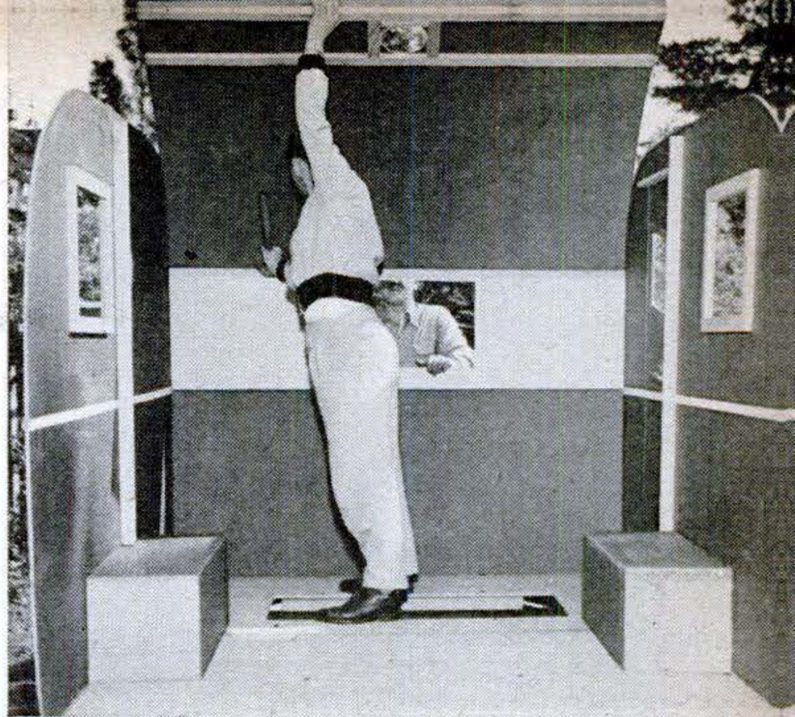
Top curves into place after side walls and front bulkhead have been attached. All seams are caulked to keep out water. Sides and top are composition board, reinforced with wood.
