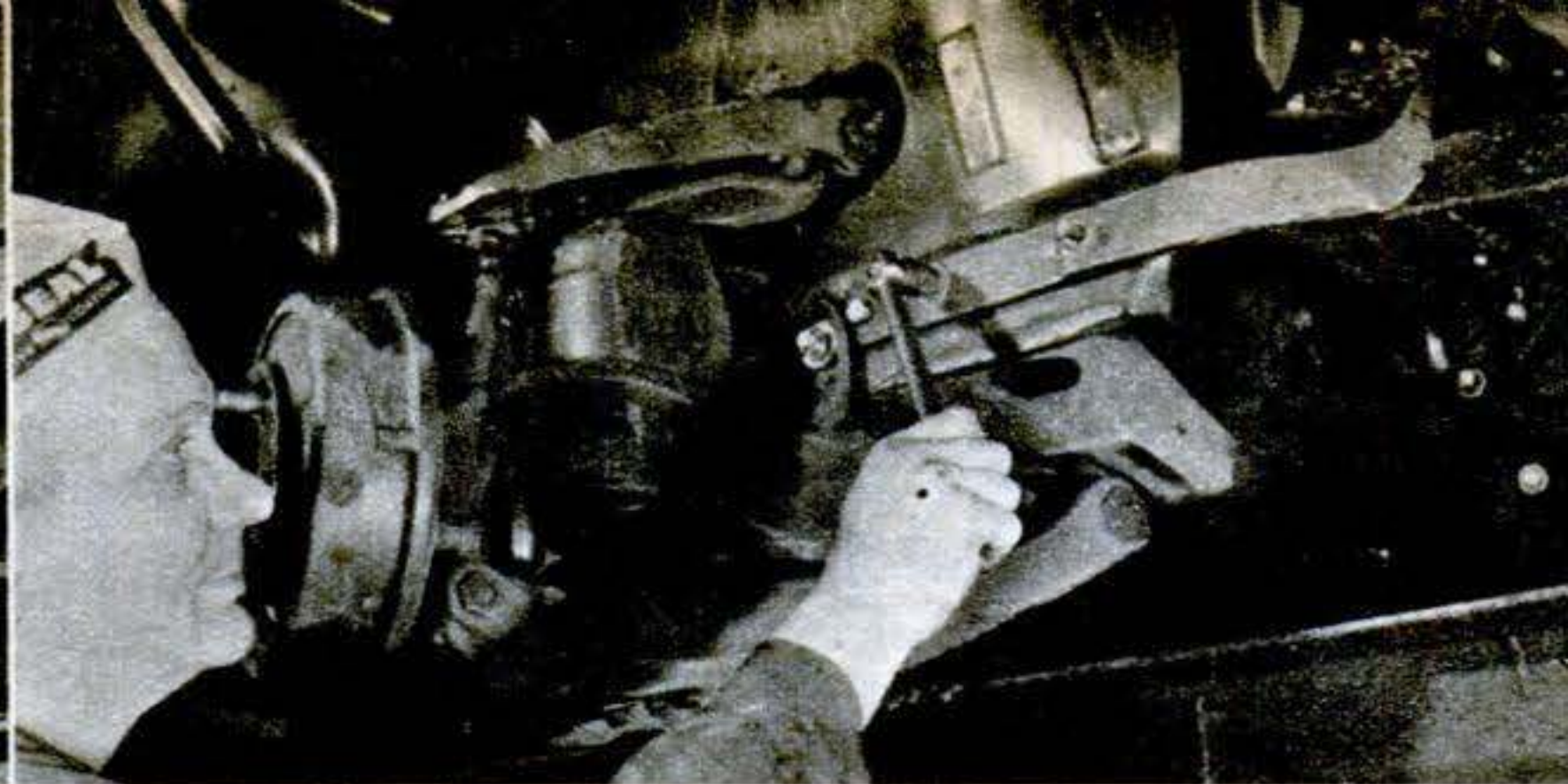
2. Body bolts must be tight, for undercoating material will cover them up. Sealed in, bolts are less likely to loosen. Note that wheels have been taken off to give more working space.
